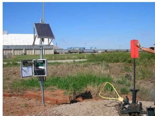
Figure 3. Solar-Powered Wayside Interface with Radio
