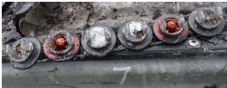
Figure 55. Module 7 valves contain material resembling nearly dried AFFF residue.
