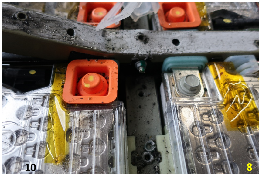
Figure 69. Clear plastic covers on each module and orange silicone-like rubber insulators were found on the terminals for each of the modules. One orange cover has been removed to show the high voltage terminal
