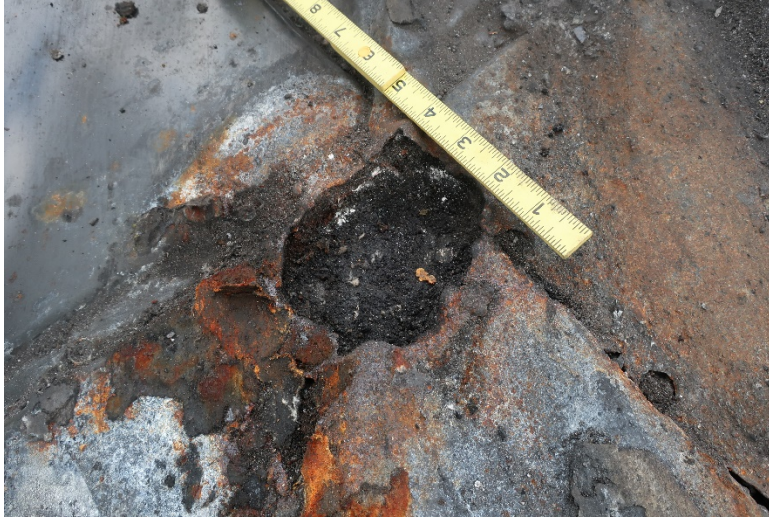
Figure 29. Close view of holes with a scale marked in inches.
