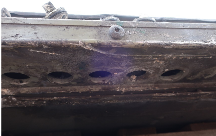
Figure 59. Module 9 vent openings.
