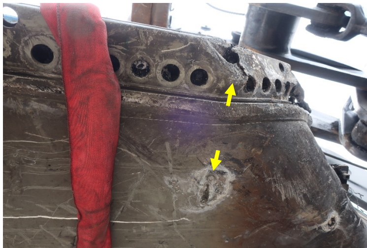
Figure 62. Module 11 vent openings. The outer edge of the buckle in the battery is along the partition between modules 11 and 13, denoted by the bolt (lower arrow) which fastens the partition internally, and spacing between the vents (upper arrow).
