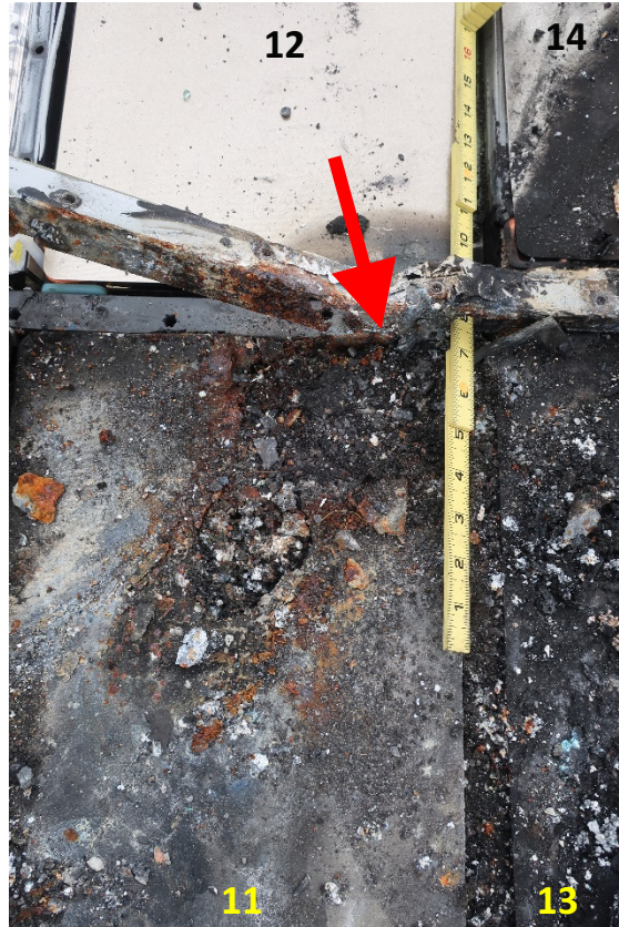
Figure 67. Close view of a hole in the mica covering module 11, the missing terminal, and surrounding damage. Numbers have been added to denote modules. The red arrow is in the same orientation as in the previous photo.
