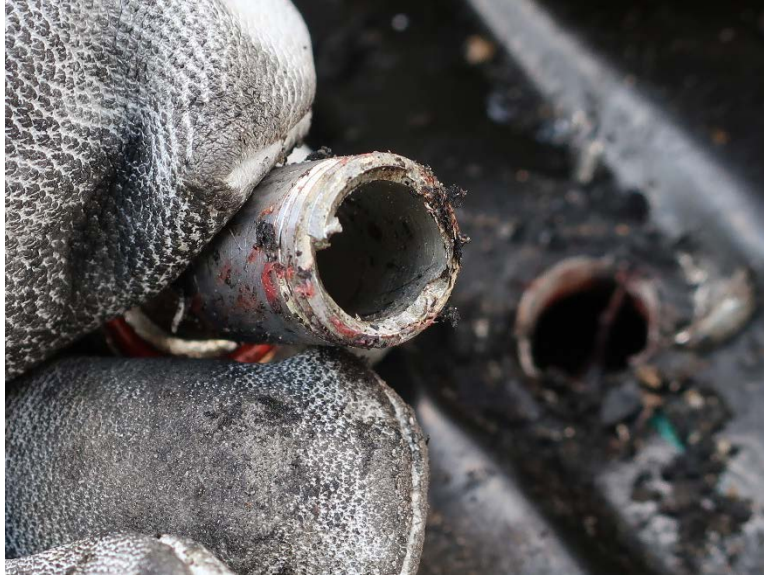
Figure 36. Fracture of a mounting bolt for the 400 VDC traction battery in gloved fingers.
