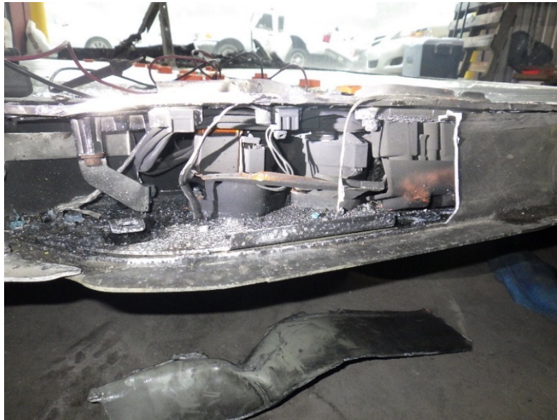
Figure 75. The end of the aluminum BMS compartment wall separated when force was used to open the top cover. This view shows the burned interior around the large contactors.
