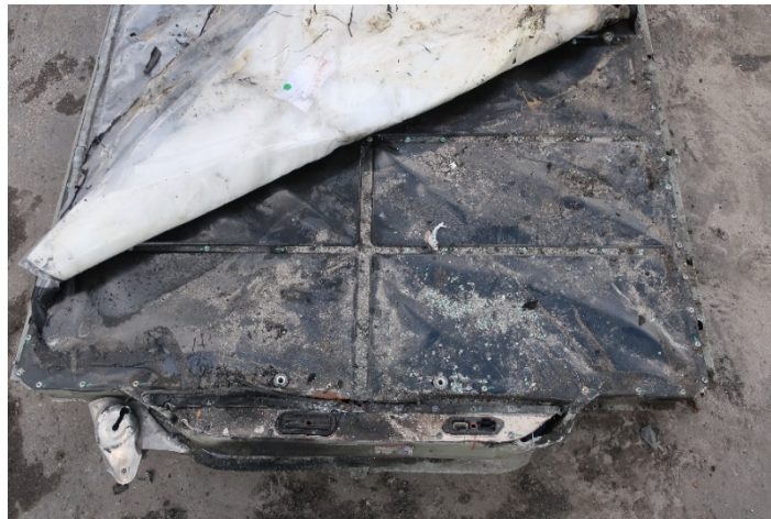
Figure 39. Rippled top steel surface of the 400 VDC traction battery after lifting insulation and water proofing layers.
