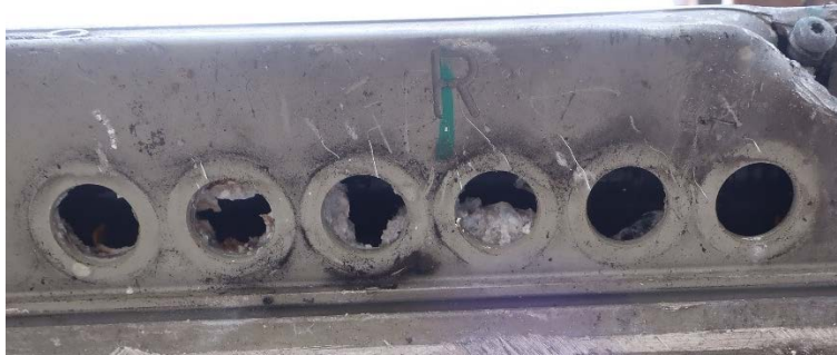
Figure 56. Dried material is visible in the open module 7 valve openings.
