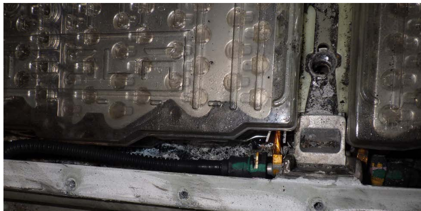
Figure 73. Outer edge of module 7, showing water droplets and light discoloration which resembled the color of dried AFFF.
