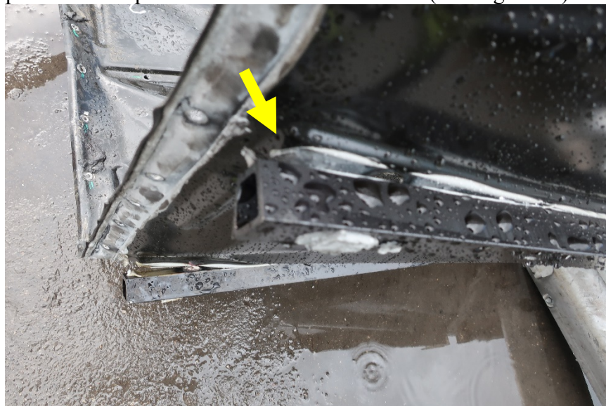
Figure 72. Outboard end of a square tube which was the upper half of a partition between modules. The arrow points to an open gap between modules. (The water visible is from a passing rain shower.)
