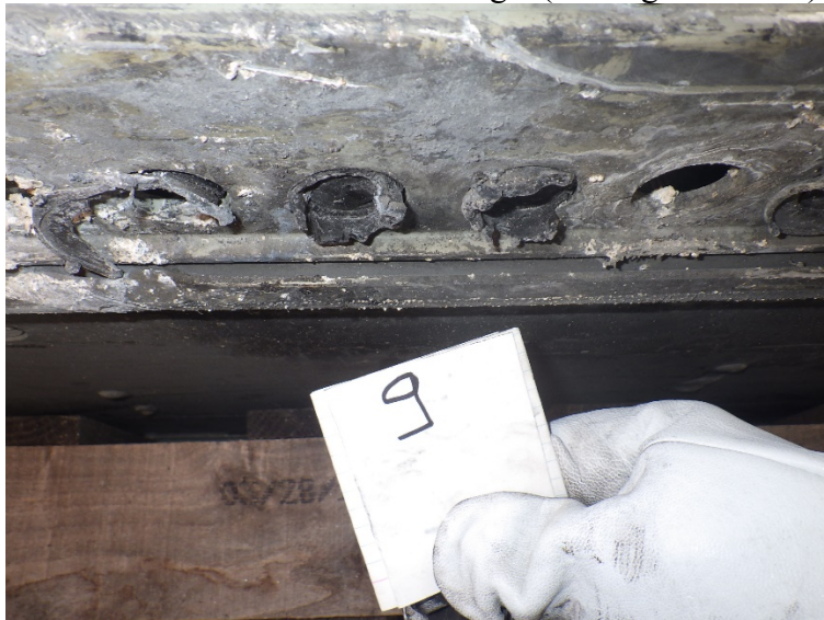
Figure 57. Module 9 valve damage prior to removal.
