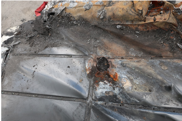
Figure 28. Closer examination found a set of oblongated holes (similar to the figure “8”) melted through the steel cover over module 11. The plastic water barrier and sheet of insulation have been removed.
