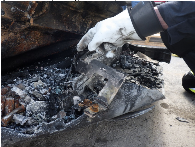
Figure 41. The photo shows the interiors of modules 13-16 after lifting the rusted battery case cover was lifted. The flat metal beneath the hand is a bus bar.
