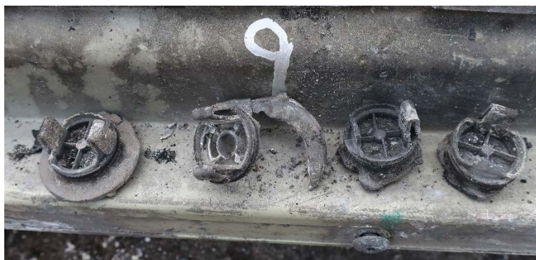
Figure 58. The four remaining module 9 valves were extensively damaged.
