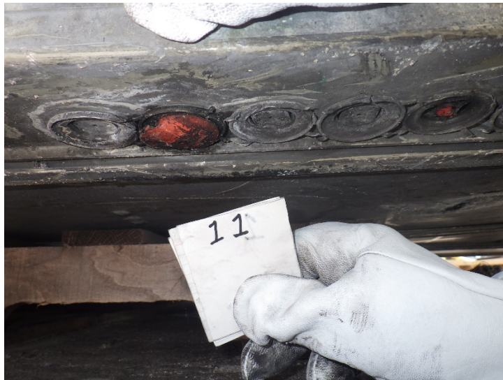
Figure 60. Module 11 valve damage prior to removal.
