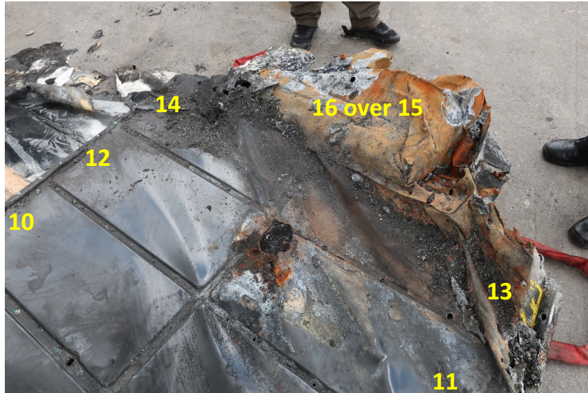
Figure 64. Forward portion of traction battery after removal of the water barrier and insulation blanket. Numbers have been added to denote modules. Note the holes at the inboard forward corner of module 11.
