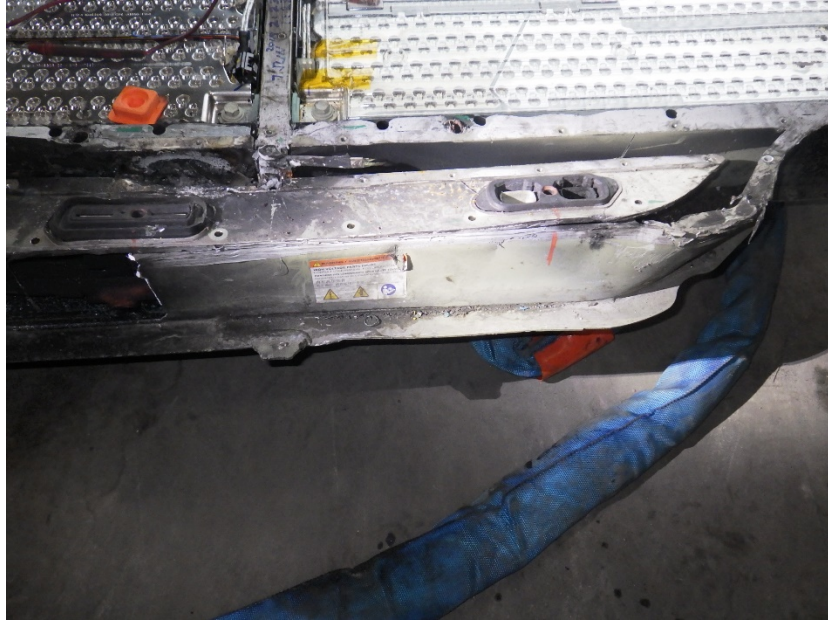
Figure 74. The BMS compartment was found with dislocated and open ends as shown. The exterior paint was had soot on the surface but was not burned.
