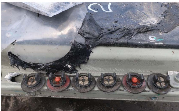
Figure 45. Module 2 valves after removal, showing module faces. Note that the valves are wet and contain tan sandy material which resembled the mica sheets covering each module, beneath the steel top of the battery case.
