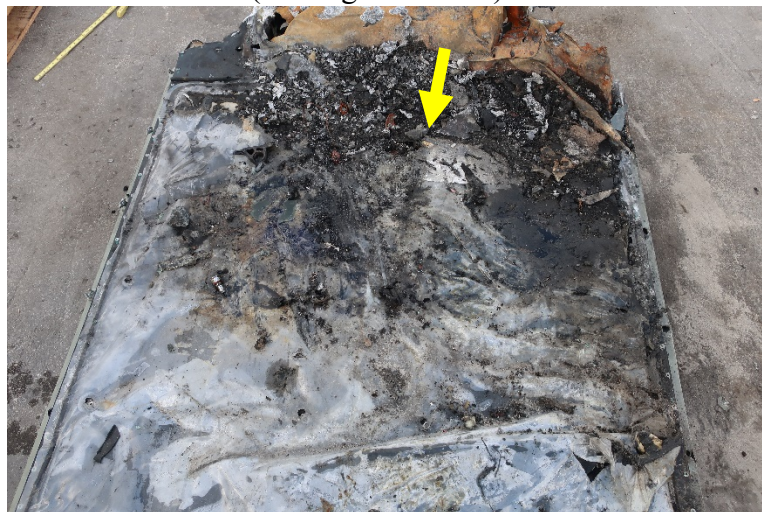
Figure 37. Insulation and plastic water liner covering forward portion of 400 VDC traction battery. The arrow points to the holes in Figures 28 and 29.
