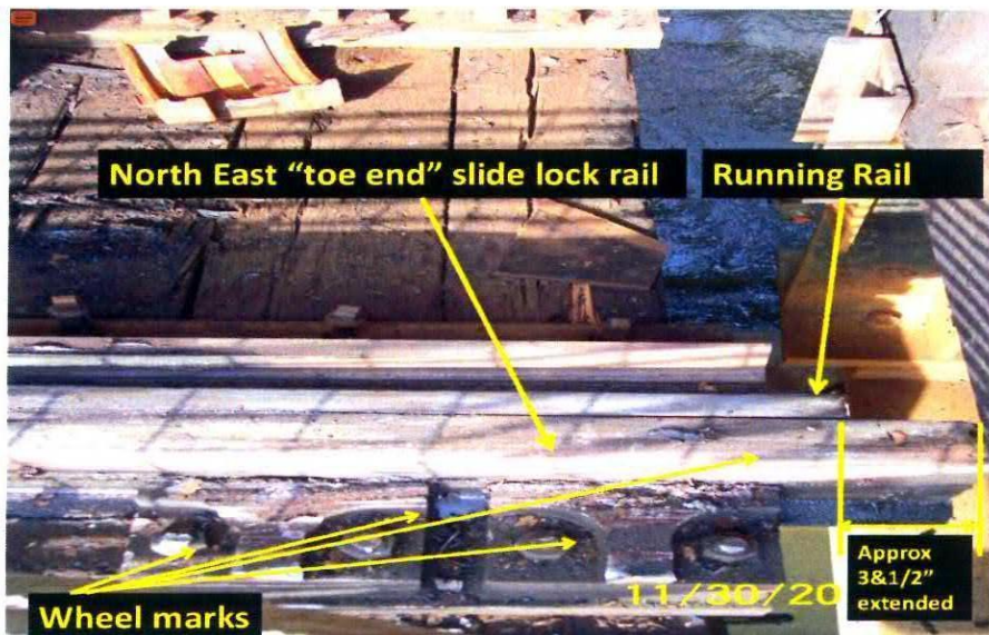
Figure 2: Bridge Slid Locks North End
