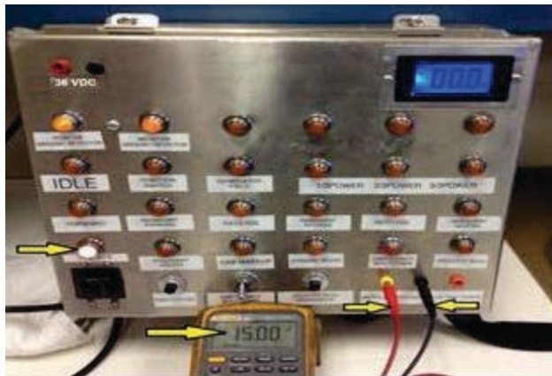
NJT Master Controller Bench Test Equipment (BTE)
