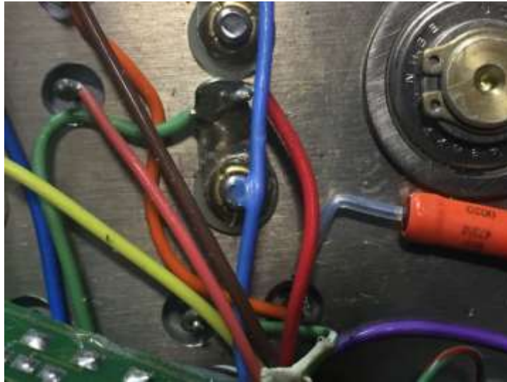
KSA 372 SN M5626 Impact damaged blue wire.
