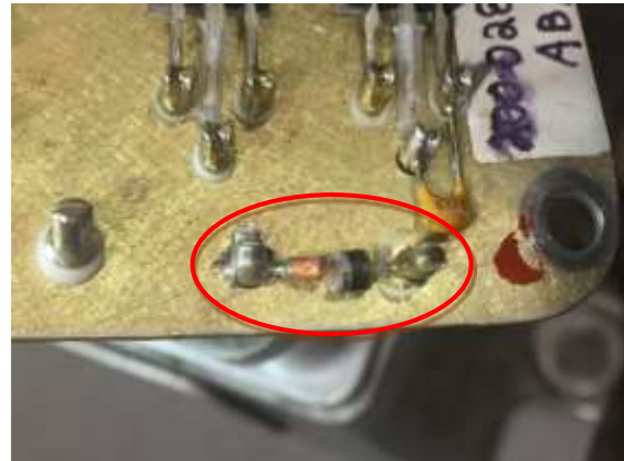
Broken diode (CR403) on the rear plate.
