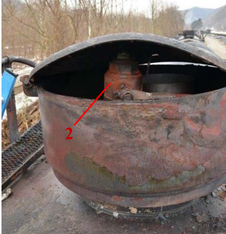
Figure 25: Liquid line upward displacement and impingement against protective housing cover.
