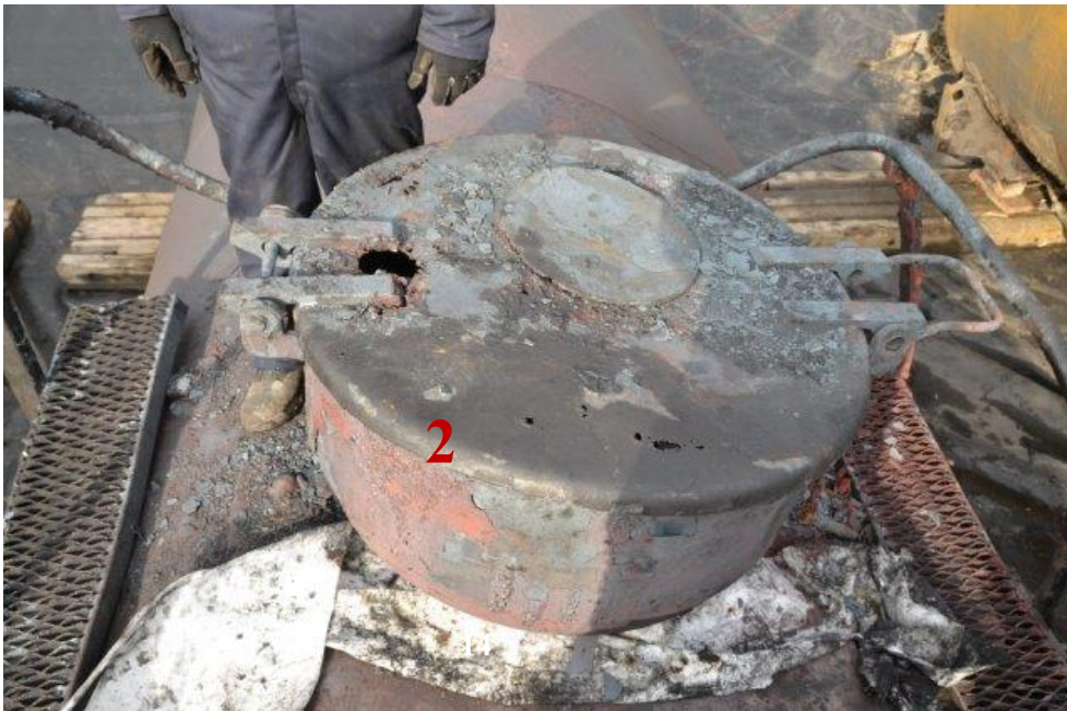
Figure 30: Top fittings protective housing cover burn-through.
