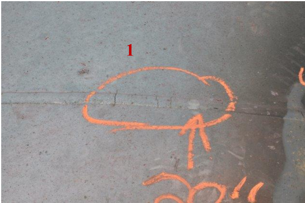
Figure 42: Close up of barrel section transverse weld cracks.
