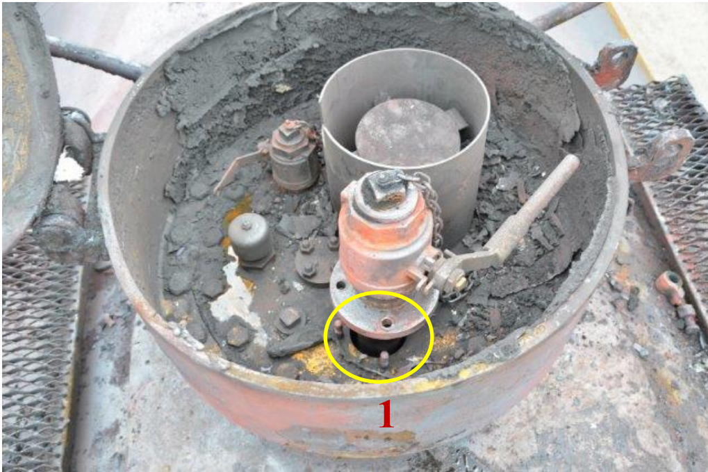
Figure 32: Liquid valve displacement upward about 5 inches, open annular space between eduction pipe and plate.
