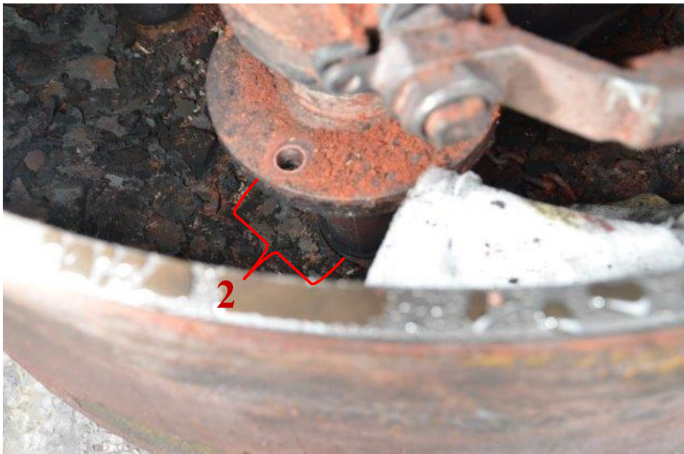
Figure 26: Liquid line valve and flange displacement, missing flange nut.
