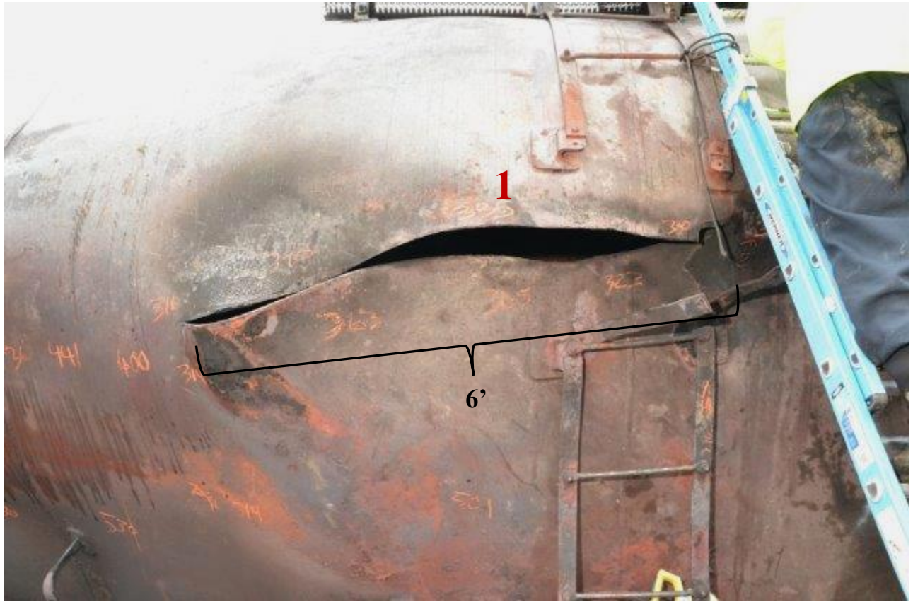
Figure 21: CBTX 741512 thermal tear with material thinning.
