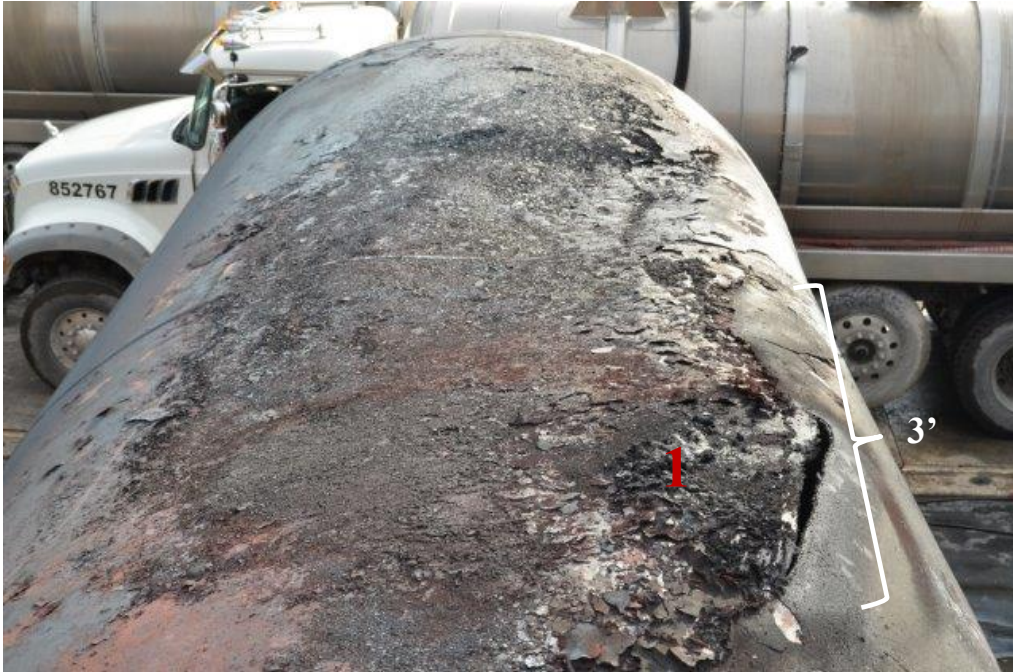
Figure 29: Thermal tear on tank top looking toward B-end, and associated thermal damage to the tank shell.
