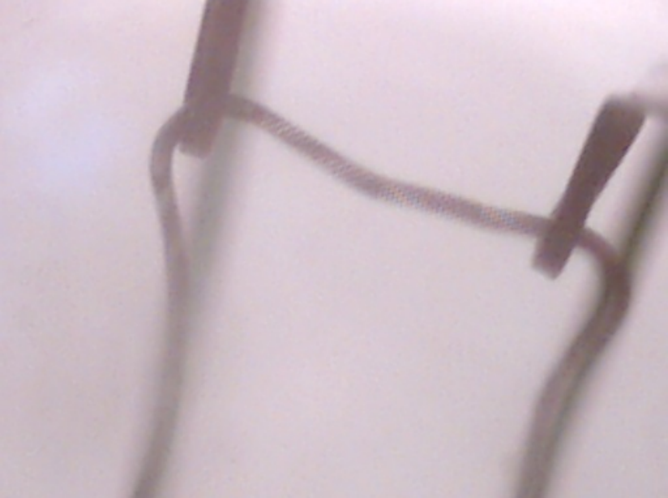
Annunciator Panel Photo 40 - Fire - Bulb B View 2
