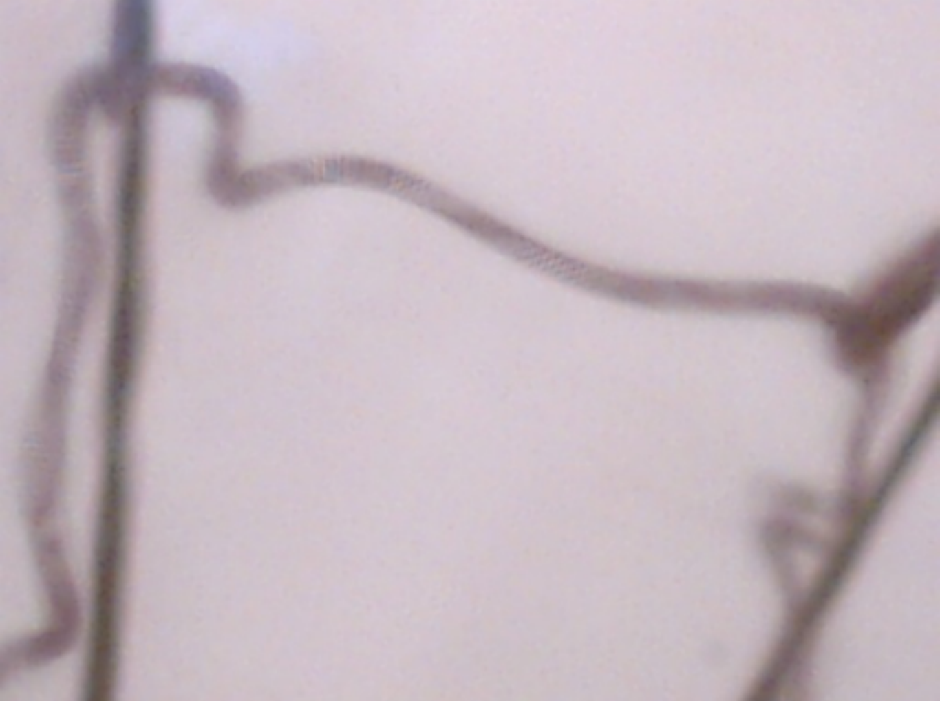
Annunciator Panel Photo 37 - Fire - Bulb A View 2
