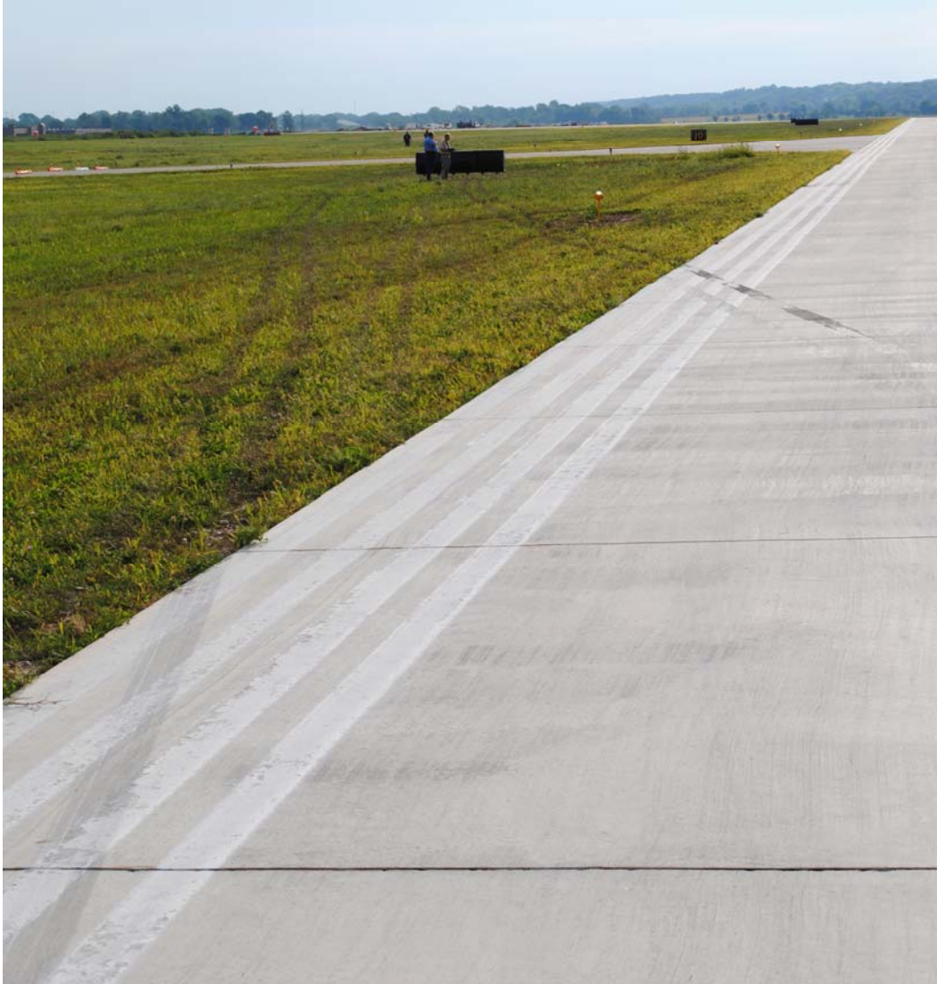
Figure 4: Close Up View of Tire Marks near Runway Departure Point
