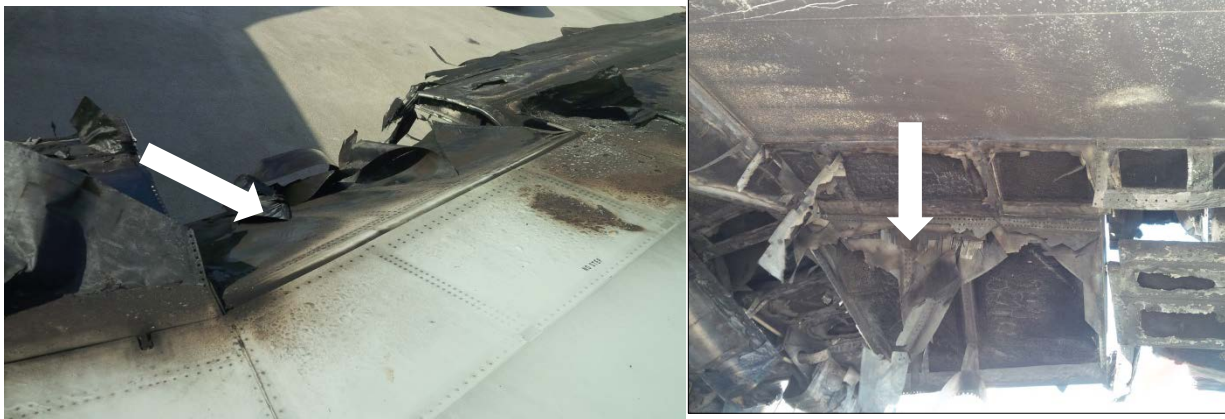
Figure 19A and 19B - Left Inboard Aileron, Top View (19A) and Bottom View (19B)
