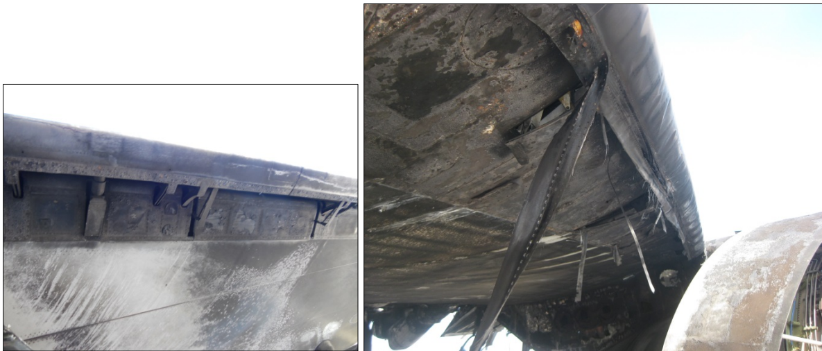
Figure 22A and 22B - Examples of Leading Edge Damage Inboard of #4 Slat (20A) and Inboard of Engine #1 (20B)
