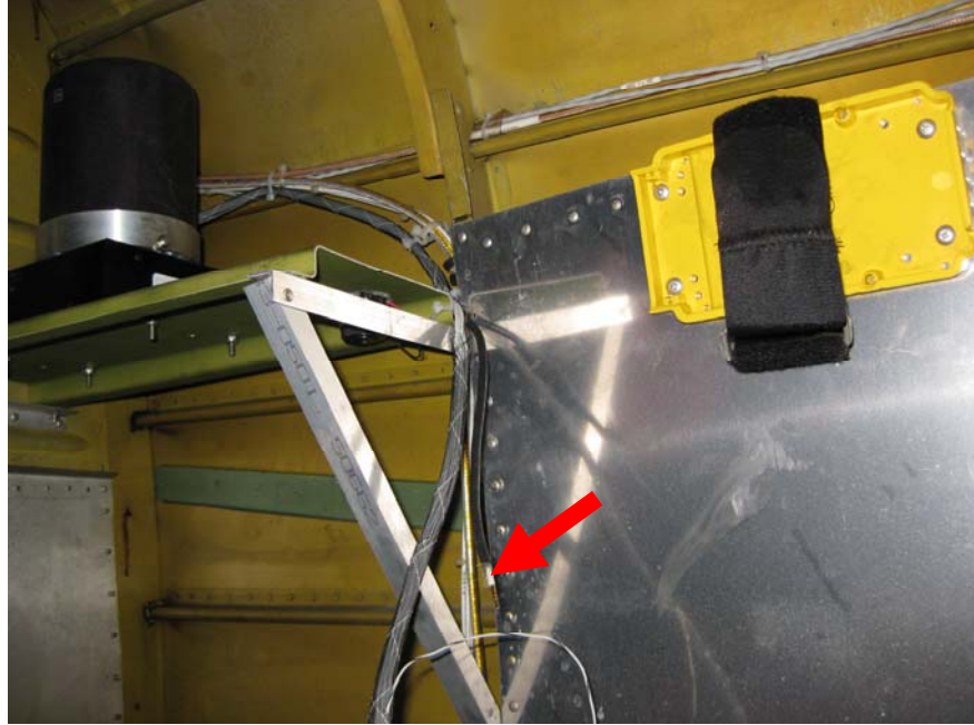
Figure 70. Empty ELT bracket in tail cone. The hook and loop fastening strap closed. To the left is forward in the airplane. The arrow points to the broken antenna connection.
