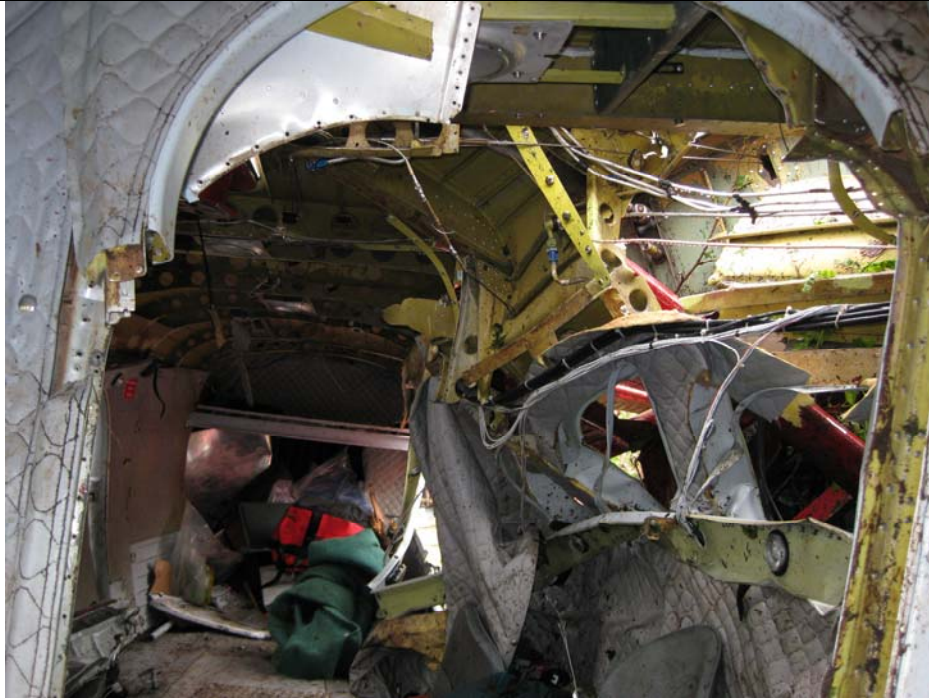
Figure 22. Prior to recovery. The left wall of the cabin can be seen displaced inward, as looking aft from the cockpit.
