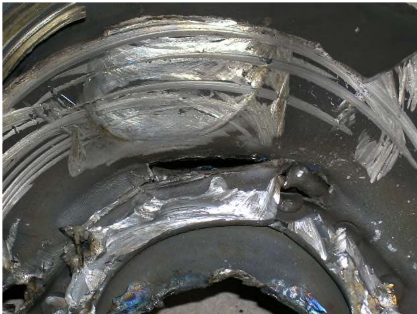
Photo No. 47 Interstage baffle downstream side, detail. Centred at the approximate 1:00 position.
