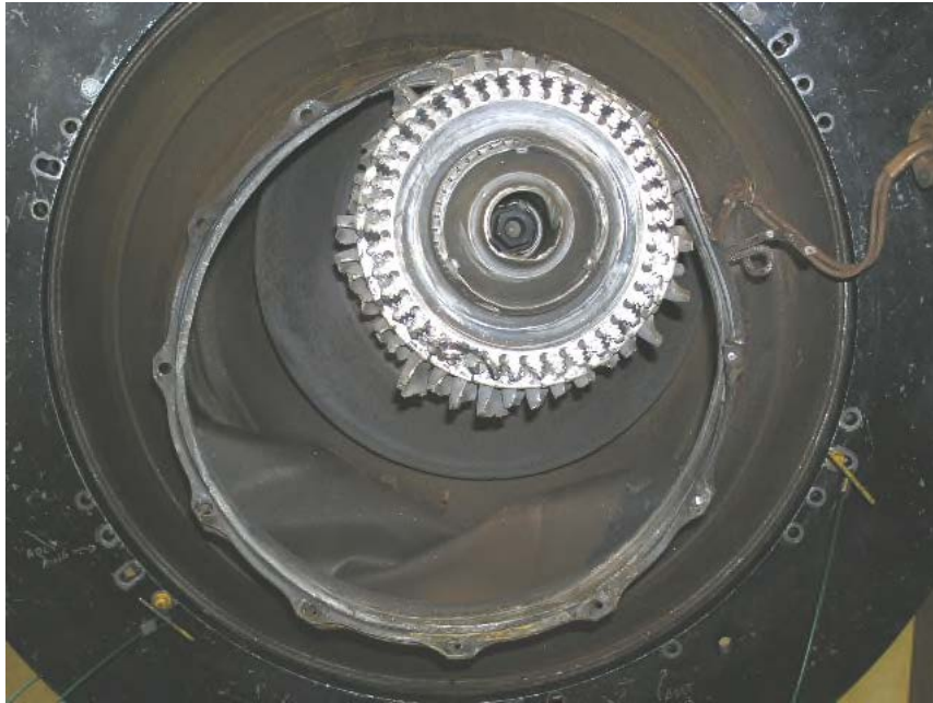
Photo No. 49 Power turbine downstream side, in-situ.
