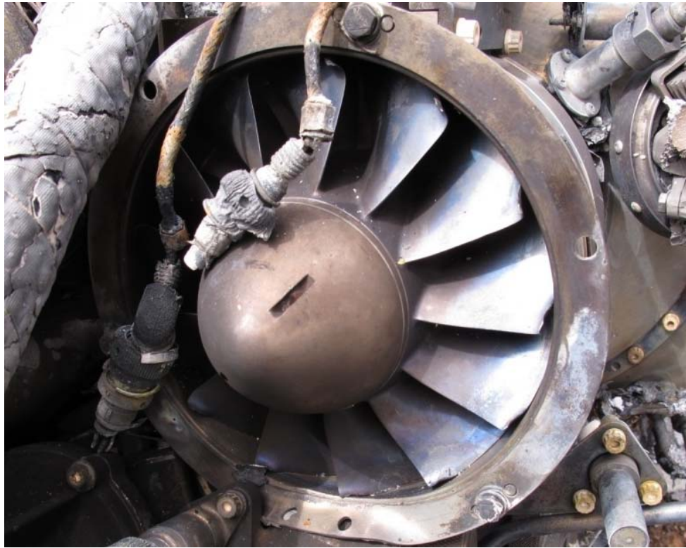
Figure 11: Photo of axial compressor and casing
