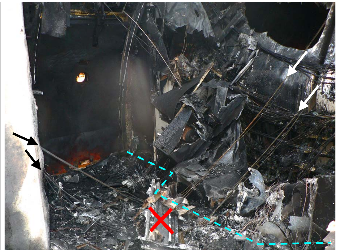
Figure 36. N799AX: The mounting for the control pulleys found on the floor of the supernumerary compartment were from the rudder, stabilizer trim, and First Officer side of the elevator system. The mounting is indicated by the red “x” at the bottom of the photograph. The arrows at the left and upper right point to the control cables. The view in this photo is from the forward left toward the aft right from the lavatory. The approximate base of the smoke wall is traced with the dashed blue line.
