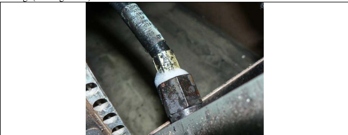
Figure 24. N799AX: Slight foaming at the right observer station hose. This slow foaming action required about a minute to produce.
