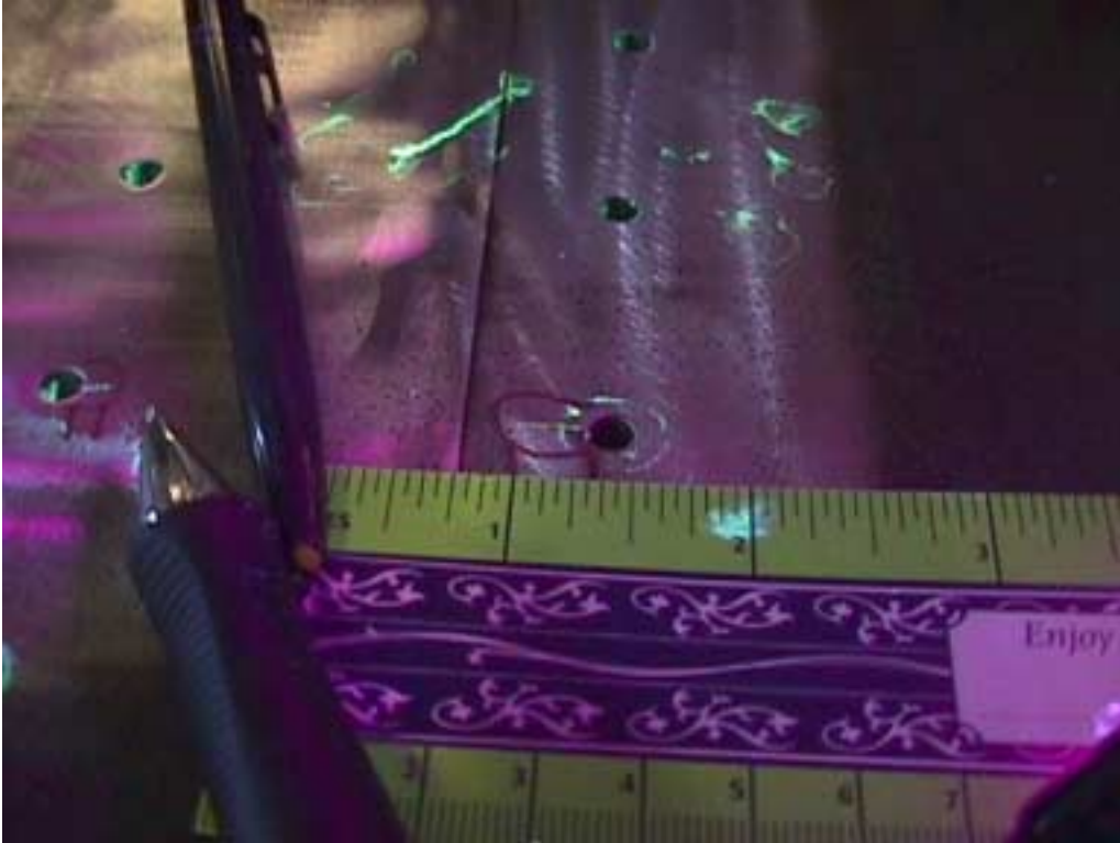
Photo 7 Crack P3 under outboard aft external doubler panel. Crack is 300'' in length. and corresponds with crack X3
