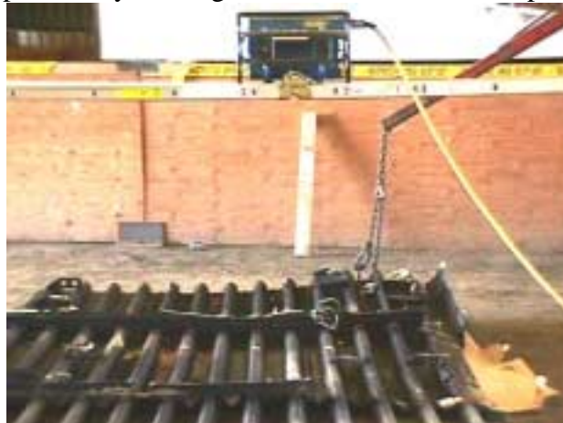
Photo-1 typical set up for x-ray of wing skins at external doubler panels
