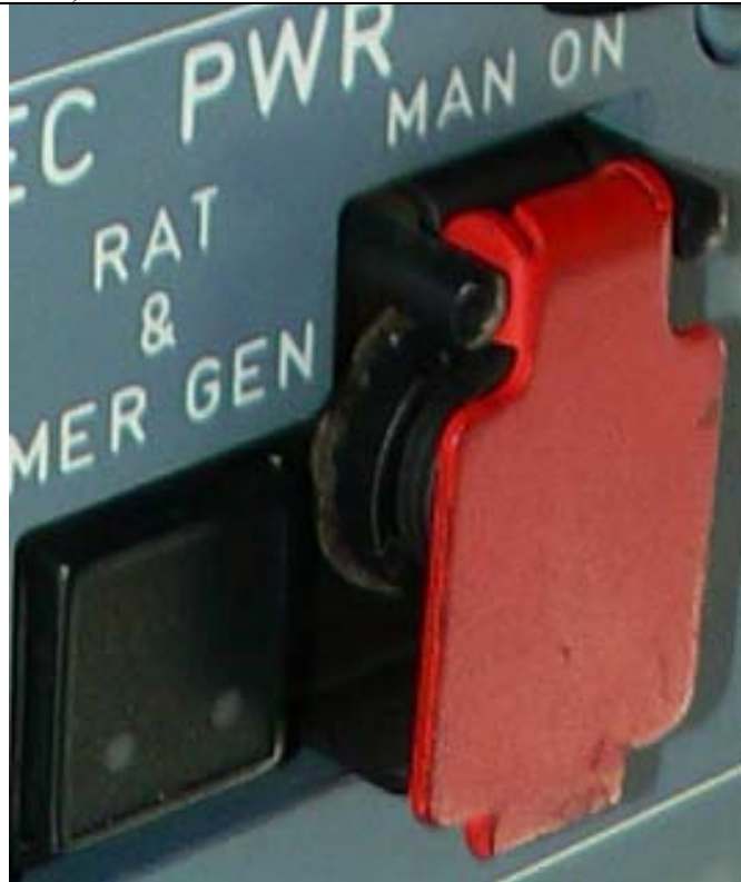
Figure 7. The edge of the MAN ON switch is visibly against the red cover, not in the depressed state. This is the EMER ELEC PWR control panel and the adjacent RAT & EMER GEN visible is not a switch, it is a fault light.
