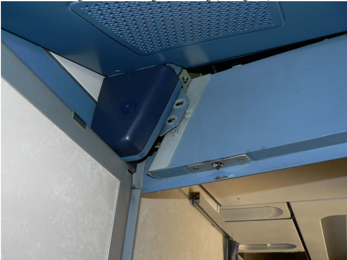
Figure 7. Panel over the cockpit door was missing screws, allowing the panel to descend
