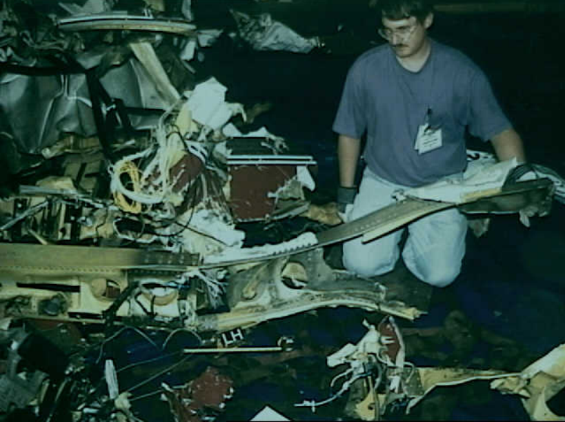
Airworthiness - Photo 11. Close-up view of the upper spar cap fitting of the wing carry-through section where it mates with the left wing spar. Note rearward direction of fractures. (NTSB-I12)
