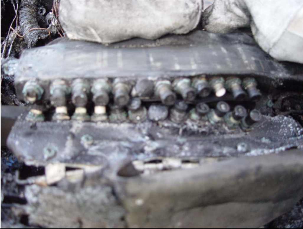
Airplane N929CD circuit breaker panel
