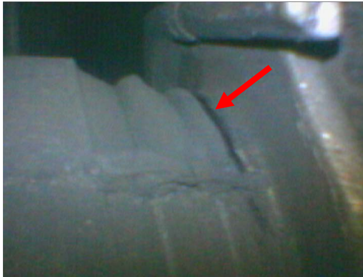
Photo 27. Suspected crack observed on the pivot bearing via video borescope. [photo courtesy of Era Helicopters]
