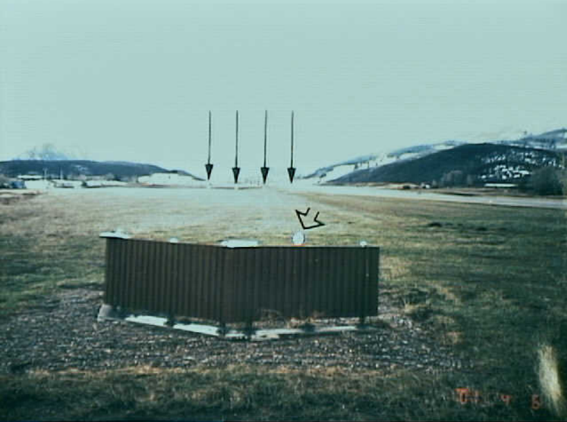
Airports/ARFF 16 - Attachment 3 - Photo 2. A close-up view looking 150 degrees magnetic showing the left REIL unit (arrow depicts lamp) and flash shielding northwest and northeast. Note the four PAPI LHA units 1,000 feet upwind (vertical arrows).
