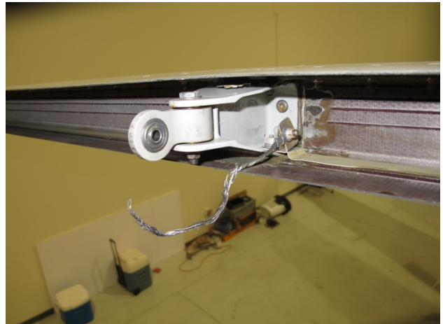
Left midspan elevator attachment fitting.
