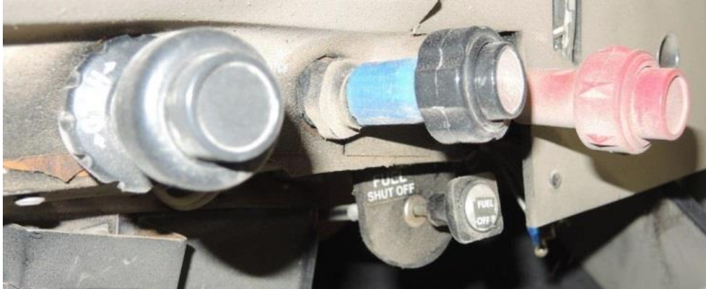
Figure 17 - Engine Controls and Fuel Shutoff
