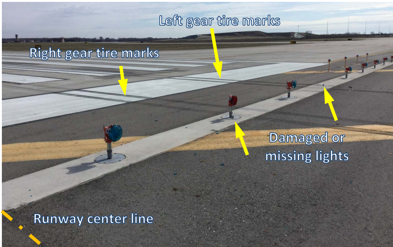
Figure 2. Threshold of runway 23L/5R and main gear tire marks on pavement.
