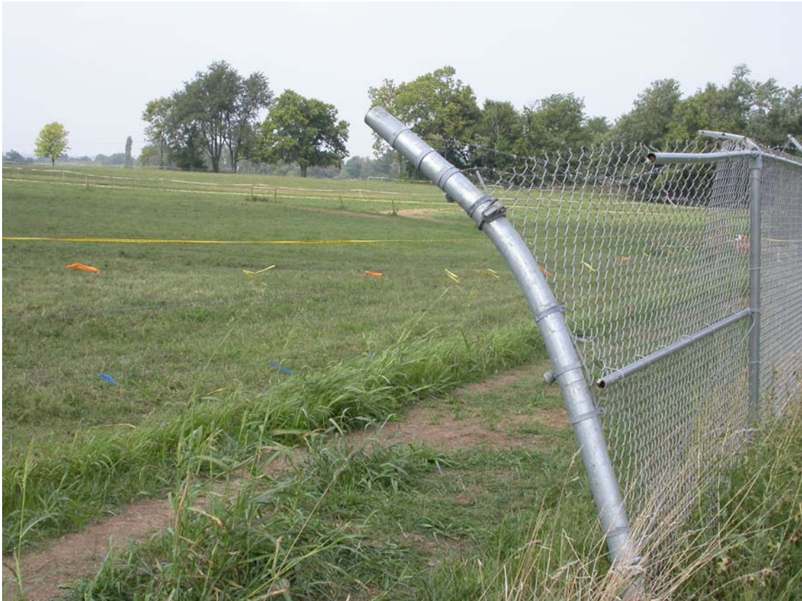
Figure 5: Perimeter Fence Gate Post Impact Damage
