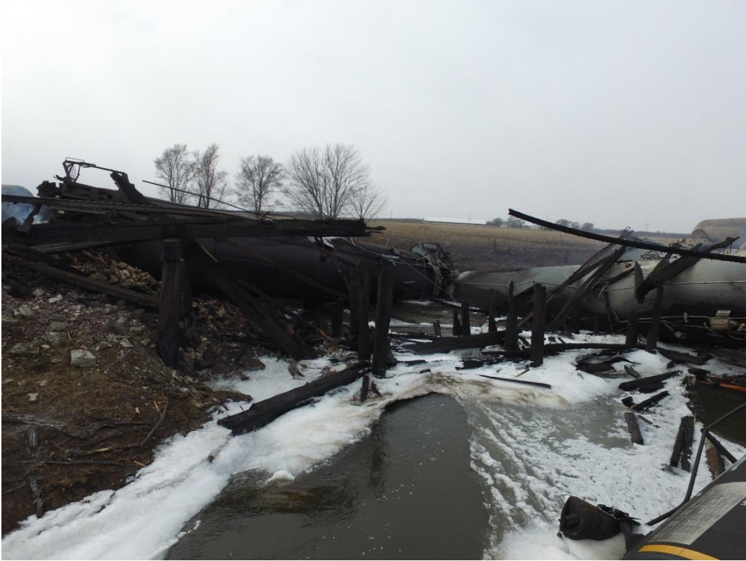
Figure 5 – Collapsed trestle looking east, viewpoint is at the original elevation of the trestle.
