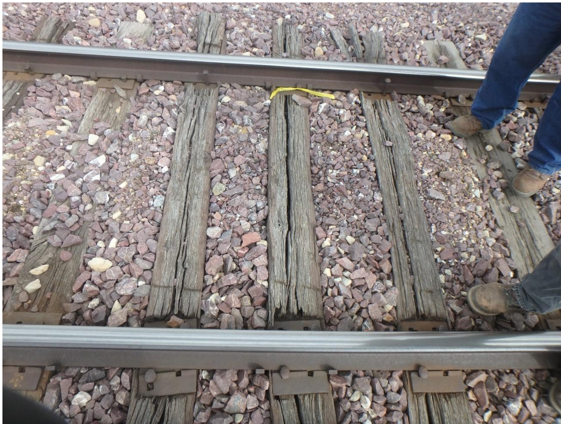
Figure 10. Split and broken crossties, that are not holding fasteners, immediately west of MP 56.9. The tie plates in the foreground have cut into the broken crossties.
