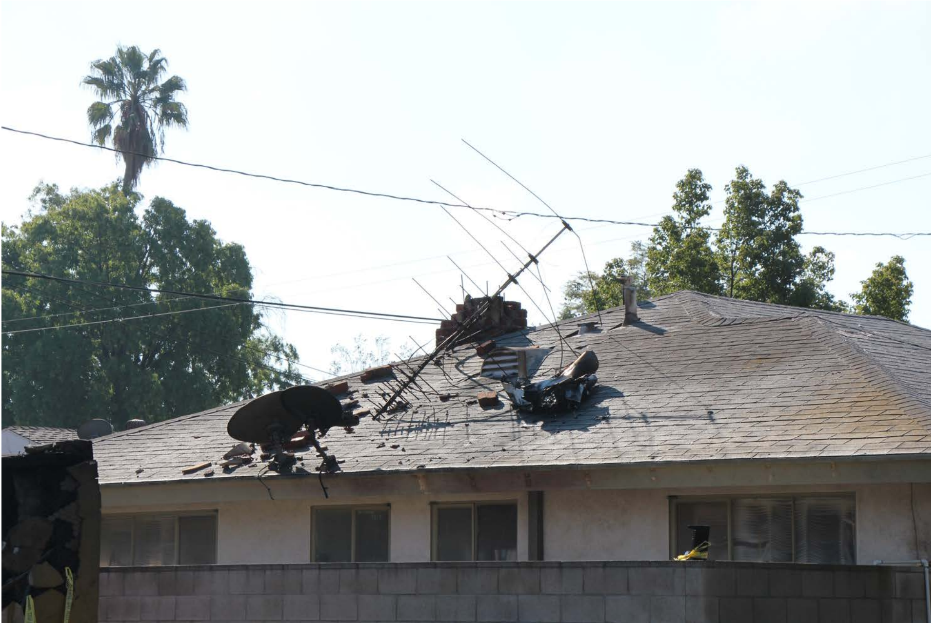
Photo 1 – View of Initial Impact Point from the North
