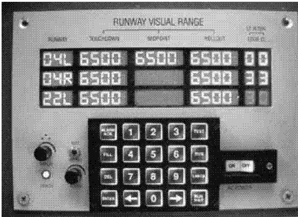
Photo 3: LIT runway visual range display
