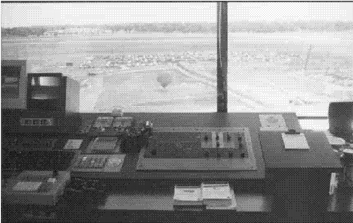
Photo 1: Little Rock runway 4R HIRL lighting control panel at LC2 position.
