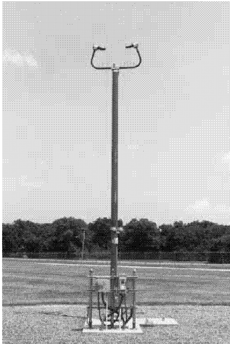
Photo 4: LIT Runway 4R RVR Sensor
