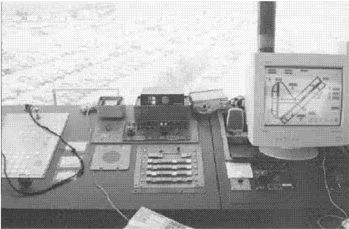
Photo 5: Approach lighting control panel at LC1 position
