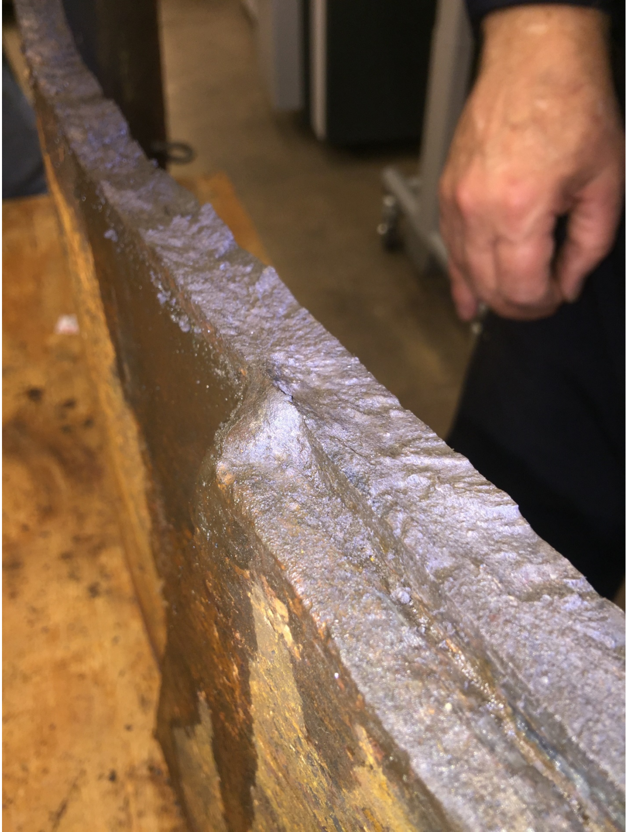
A-L cradle pad fillet weld termination and crack initiation location
