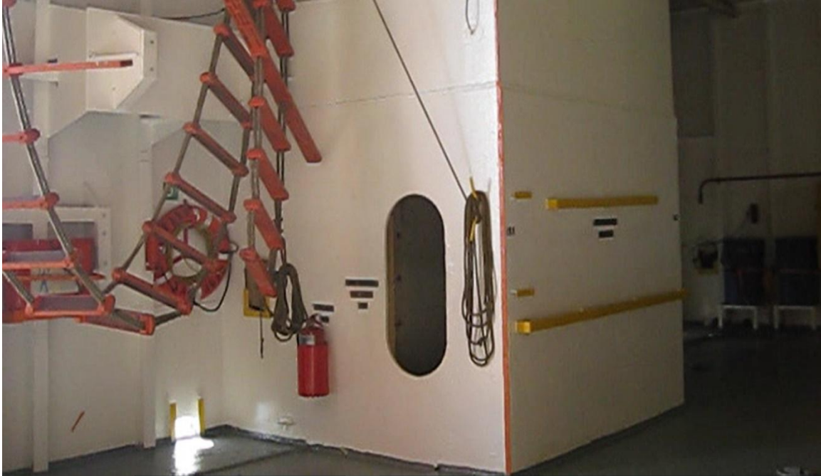
Figure 6-11: Hold 3 aft ventilation exhaust trunk with racking bulkhead, frames 159-162 starboard, 2 nd deck. Screen capture from video taken September 2008 provided by Tote, Inc.
