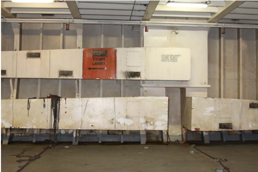
Figure 6-13: Ventilation supply plenums inside Hold 3, frames 141-144 port, 4 th deck (tanktop, innerbottom). Photo of sister vessel EL YUNQUE. USCG photo.
