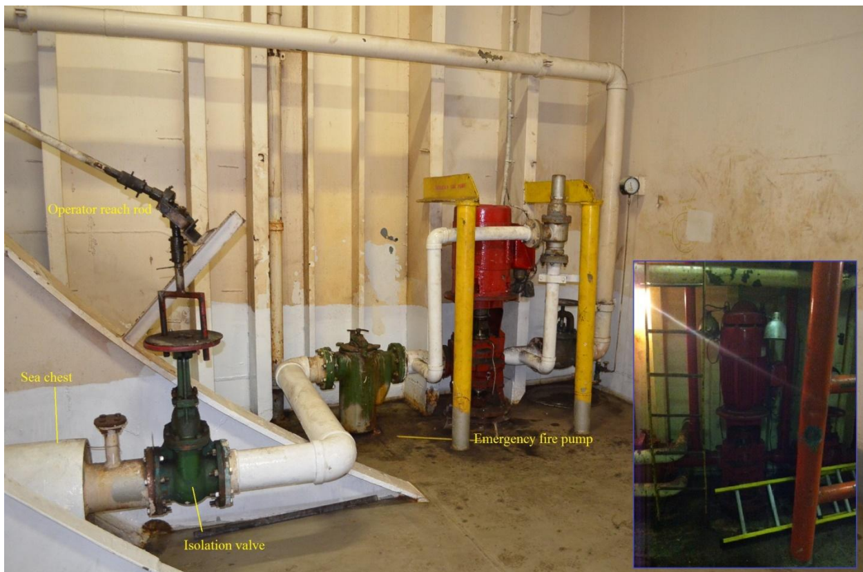
Figure 6-7: Emergency fire pump station in Hold 3, aft starboard 4 th deck (tanktop, innerbottom), showing the sea chest, isolation valve, and manual remote operator on sister vessel EL YUNQUE (EL FARO similar but not identical). Inset photo shows part of the arrangement onboard EL FARO. USCG photo with Tote, Inc. photo inset.
