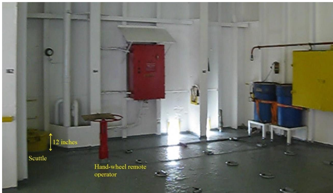
Figure 6-6: Hold 3 (also called Hold D) starboard personnel access scuttle on the 2 nd deck at frame 163. Note that the scuttle opening is 12 inches above the deck. The hand-wheel remote operator for the emergency fire pump sea-chest isolation valve is also shown. Screen capture from video taken aboard EL FARO September 2008 provided by Tote Inc.
