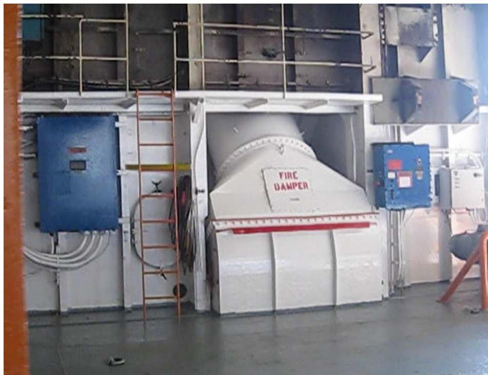
Figure 6-12: Hold 3 ventilation supply fan and fire damper enclosure, frames 141-144 starboard, 2 nd deck. Screen capture from video taken September 2008 provided by Tote, Inc.
