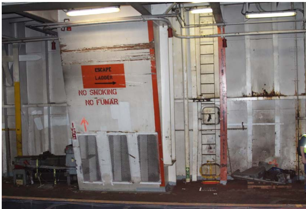
Figure 6-14: Ventilation exhaust intake plenum inside Hold 3, frames 159-162 starboard, 3 rd deck. Hold 3 starboard scuttle personnel access ladder and remote operator rod for the emergency fire pump suction valve (sea-chest isolation) are shown on the right. Photo of sister vessel EL YUNQUE. USCG photo.
