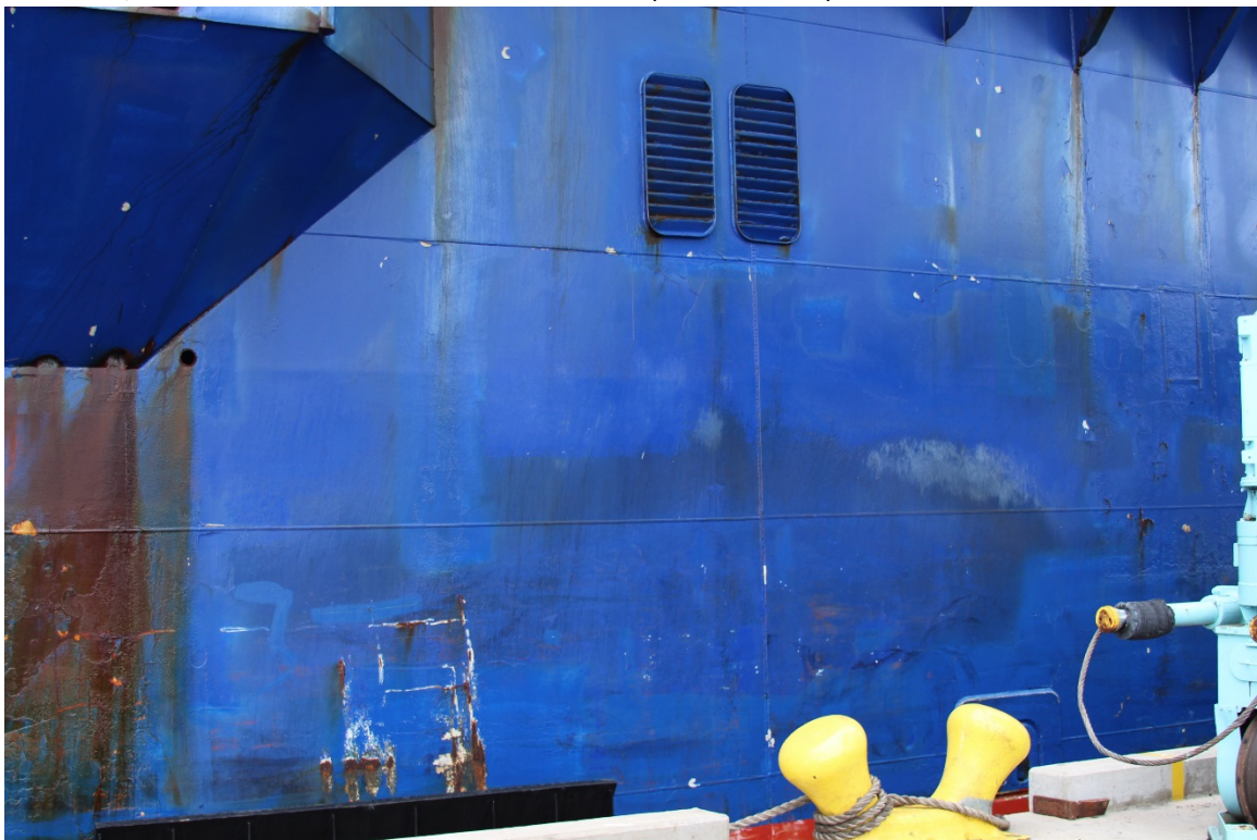
Stbd Side, 3 hold forward Exhaust louvered vents (two at fr 135)
