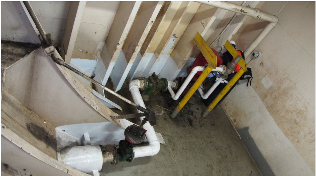
No. 3 Hold, view from Stbd Aft Corner above Emergency Fire pump system (looking Port and aft)
