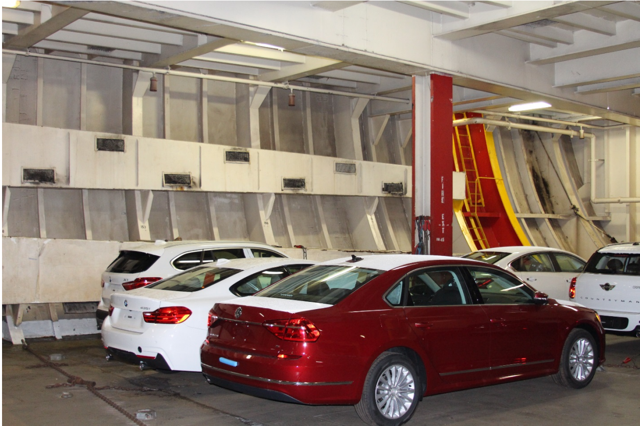
No. 3 Hold, view from center of hold looking Stbd and Aft at inlet vents, Ladder and E-Fire pump area
