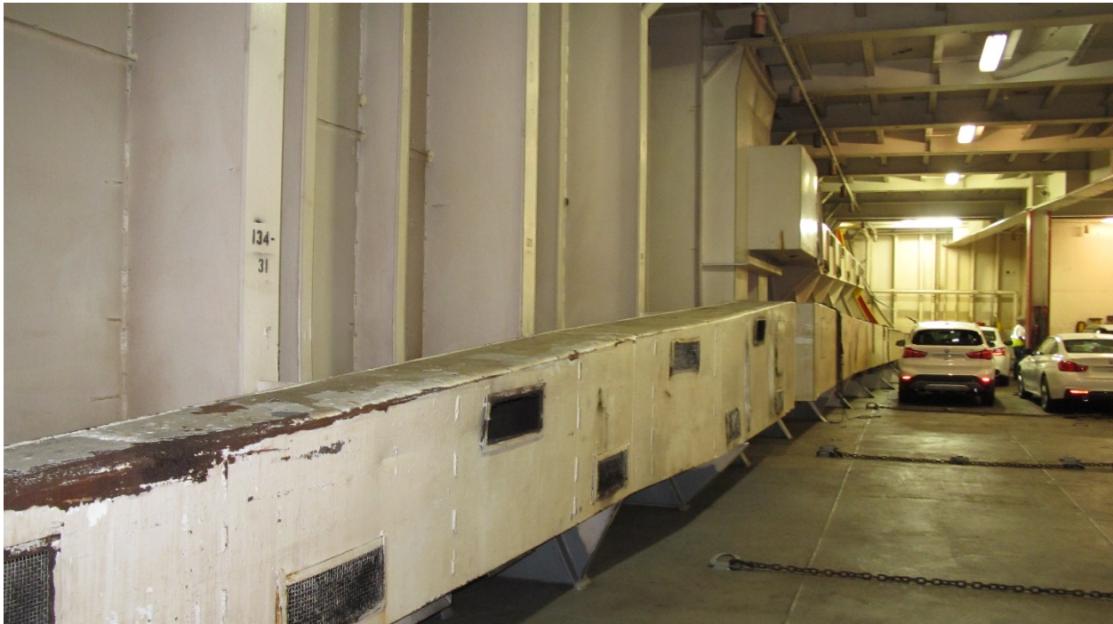
No. 3 Hold, view from fwd stbd corner looking aft (inlet ventilation ducts)
