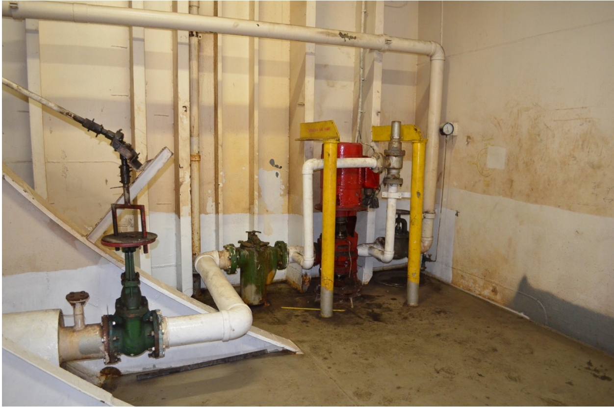
No. 3 Hold, view from Stbd Aft Corner looking Port and Aft at Emergency Fire pump system
