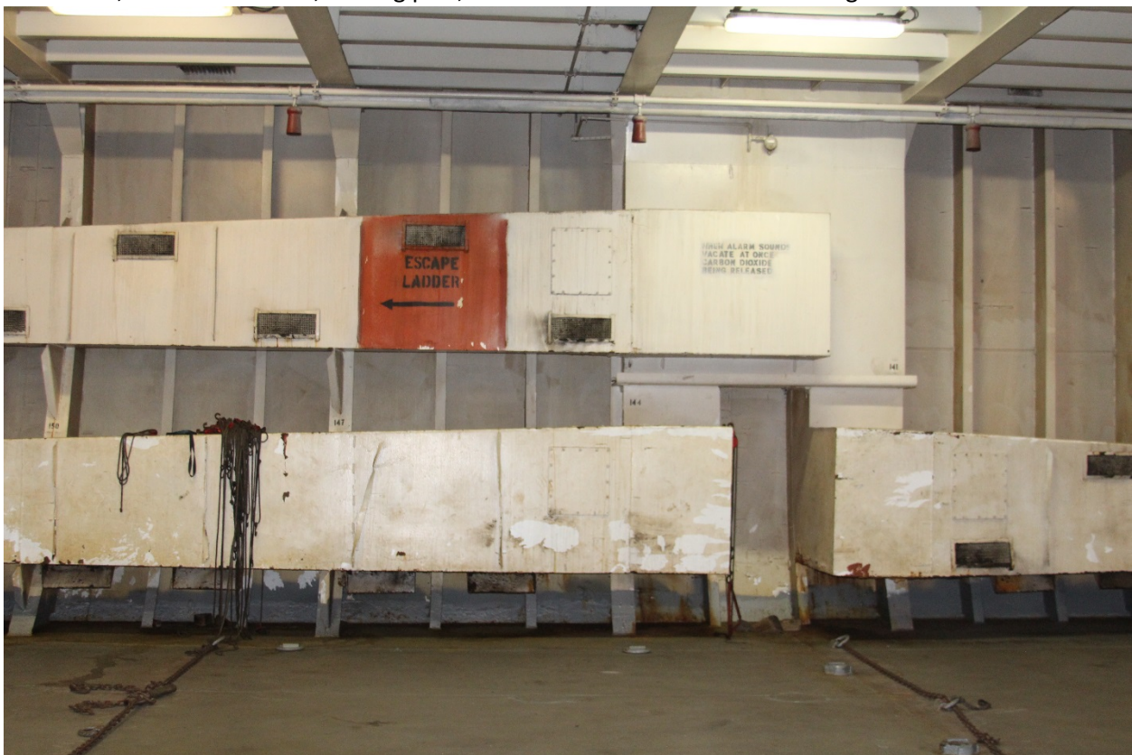
No. 3 Hold, view from center, looking port, of Port Side inlet ventilation ducting
