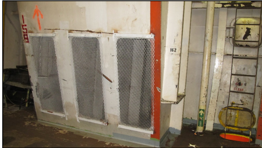
4 5 Figure 32. El Yunque , cargo hold 3, natural exhaust ventilation inlets, tween deck frames 158- 6 162. (Photo from December 2015)
