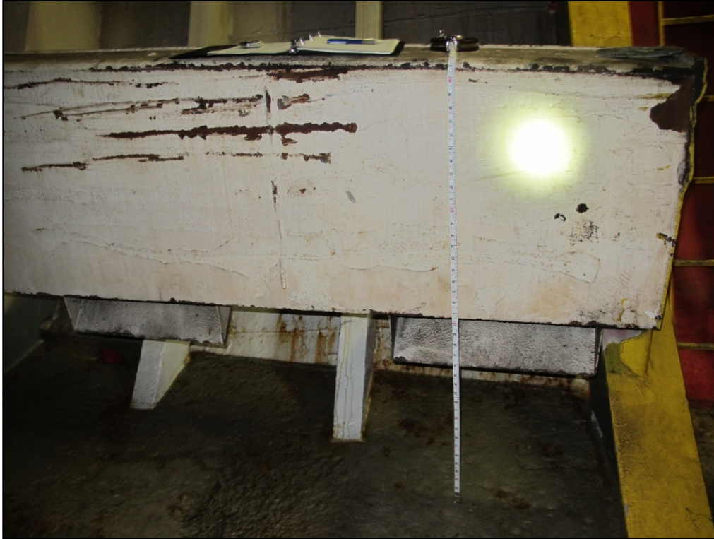
1 2 Figure 29. El Yunque , hold 3 starboard, aft, horizontal supply ventilation trunk end at fame. 162. 3 Trunk bottom 24 inches off tanktop, registers 16 inches off tanktop. (Photo from September 2016)
