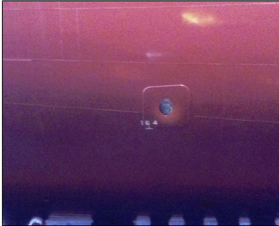
1 2 Figure 18. Penetration of sea chest for El Faro 's emergency fire pump, viewed from exterior. 3 (TOTE photo from December 2013 drydock)
