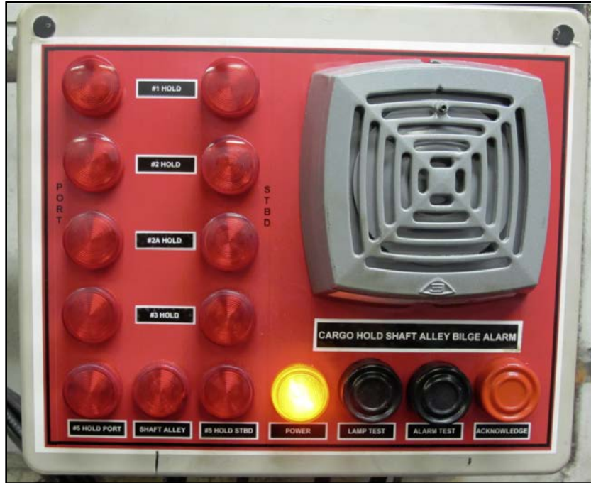
1 2 Figure 22. El Yunque bilge alarm panel on engine room control flat. (Photo from September 2016)
