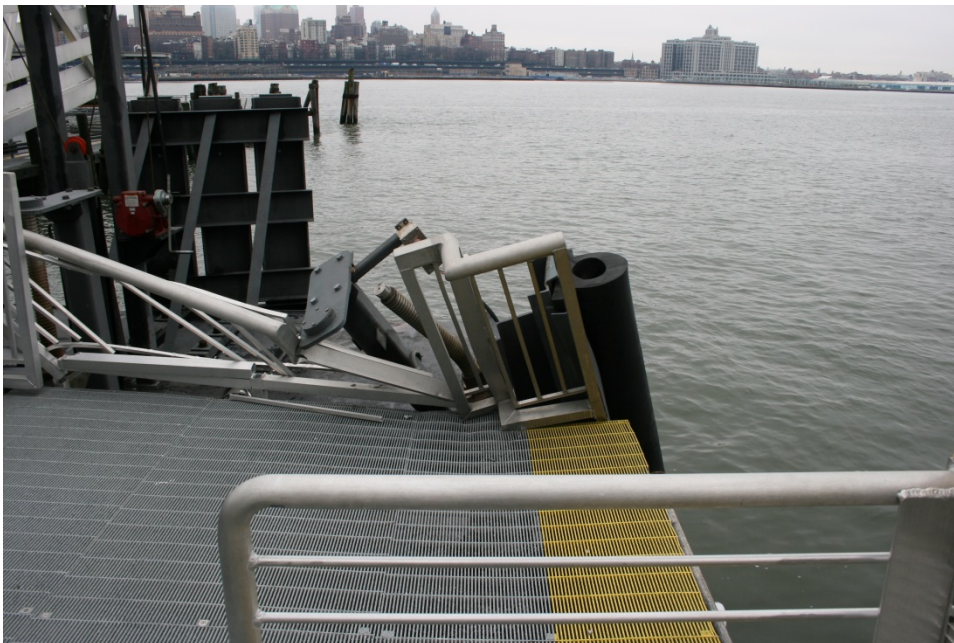
Figure 15. Damage to fender, jackscrew, and platform
