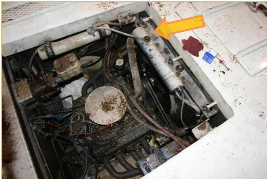
Figure A-2- 3. View of forward part of engine compartment, DUKW 34 . Gold arrow indicates missing pressure cap at surge tank.
