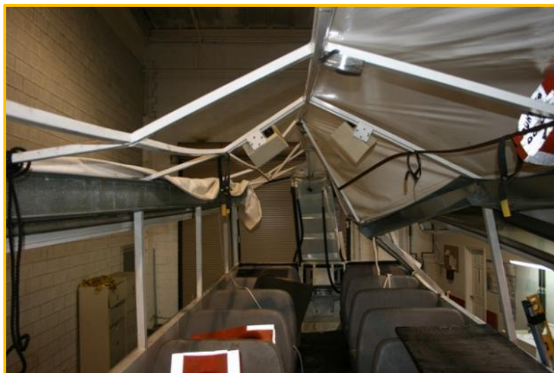
Figure 7. View of damage to canopy of APV from inside the cabin, looking aft.
