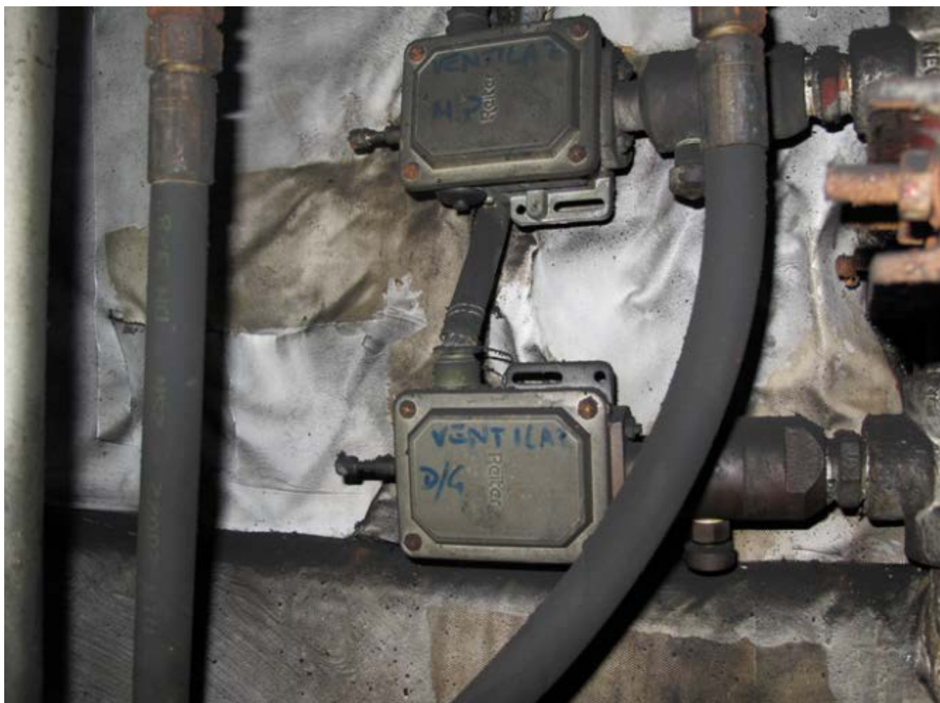
Figure 16. Photograph of ventilation control solenoids.
