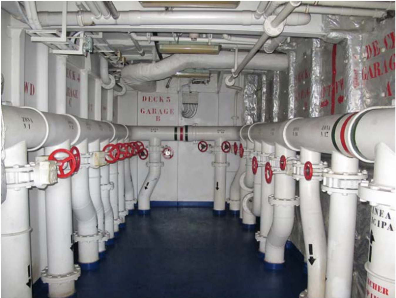
Figure 20. Overall photograph of water drencher system control station.
