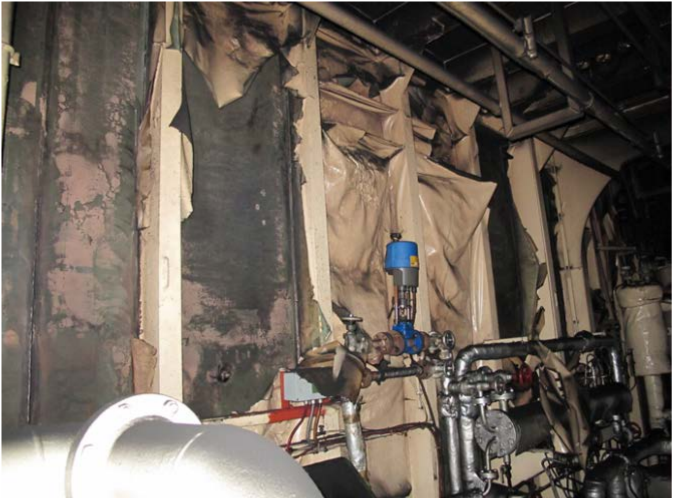
Figure 32. Photograph of bulkhead between main engine room and auxiliary engine room (auxiliary engine room side).
