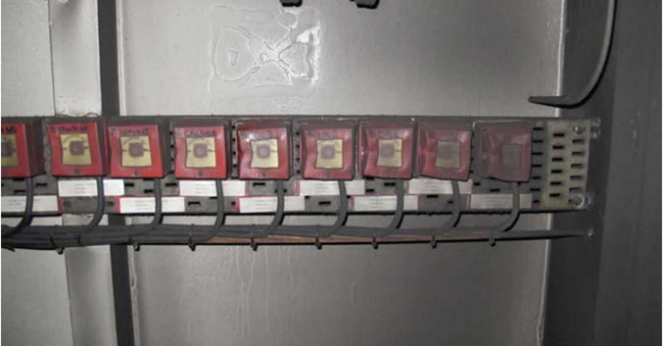
Figure 19. Photograph of water mist remote activation panel in the AC machinery room.
