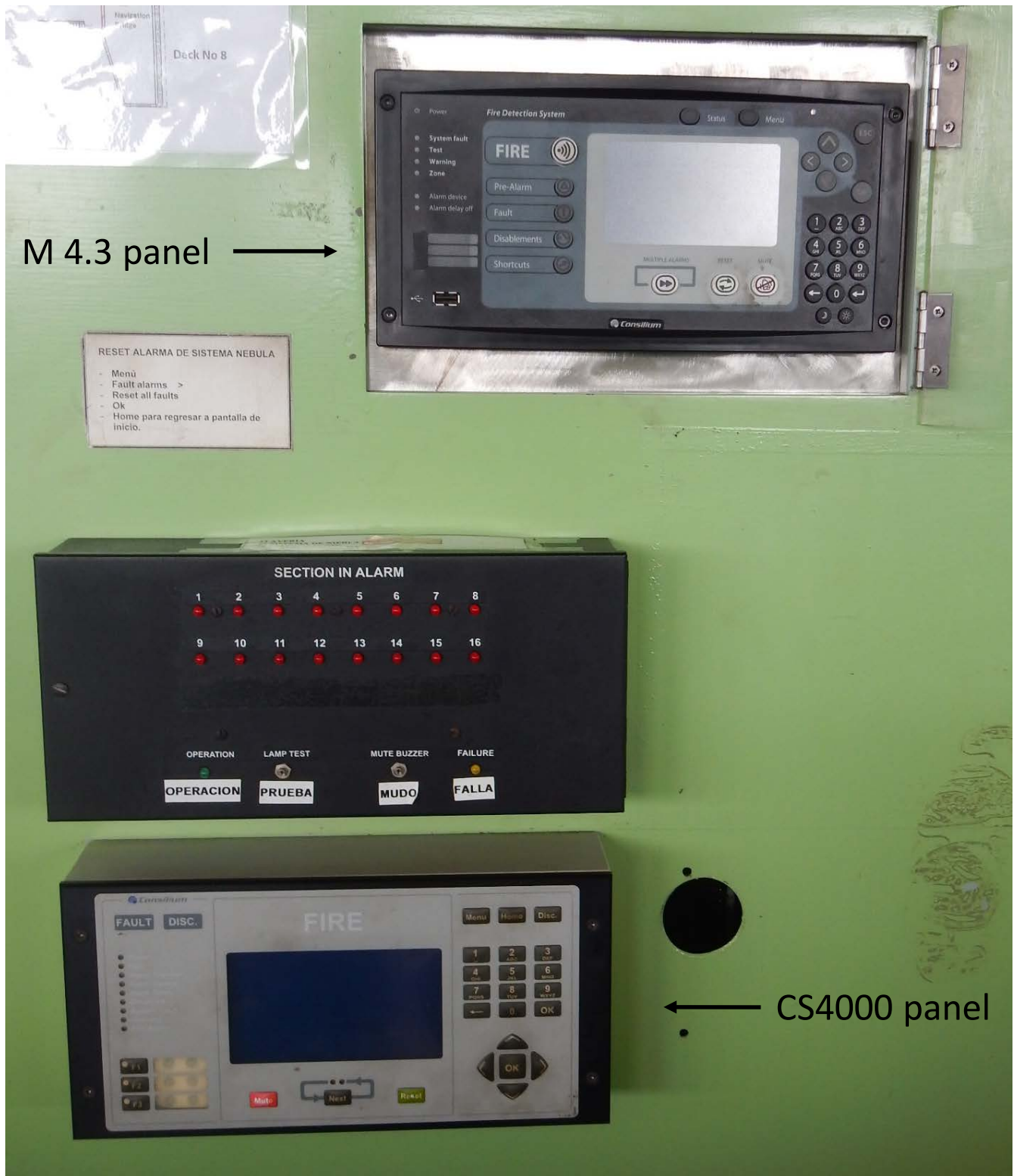
Figure 4. Photograph of fire detection system panels on the bridge.
