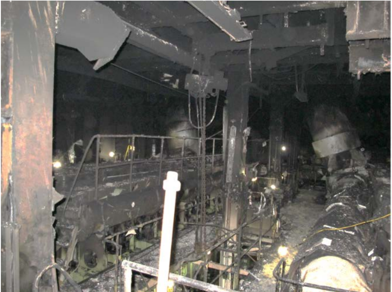
Figure 28. Overall photograph of upper deck of main engine room looking from forward to aft. The port main engine is on the right of the photograph. The starboard main engine is on the left.
