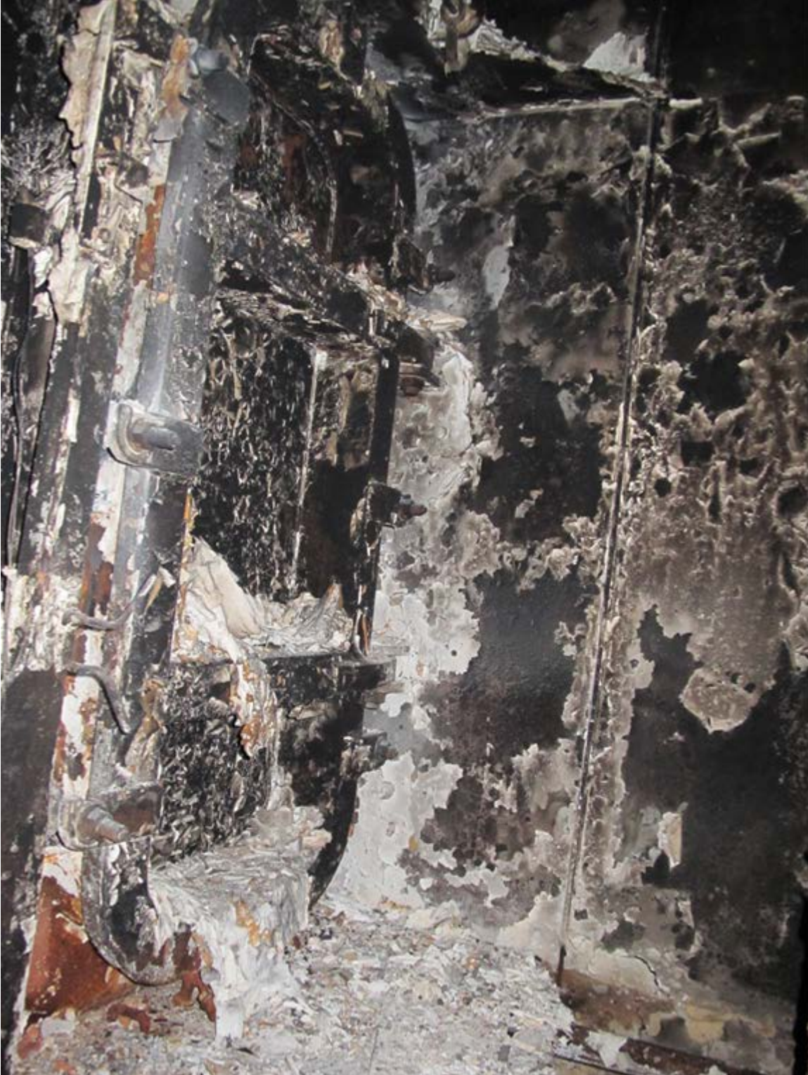
Figure 36. Photograph of the interior of the port fuel bunker station. The side shell door can be seen at the left of the photograph.
