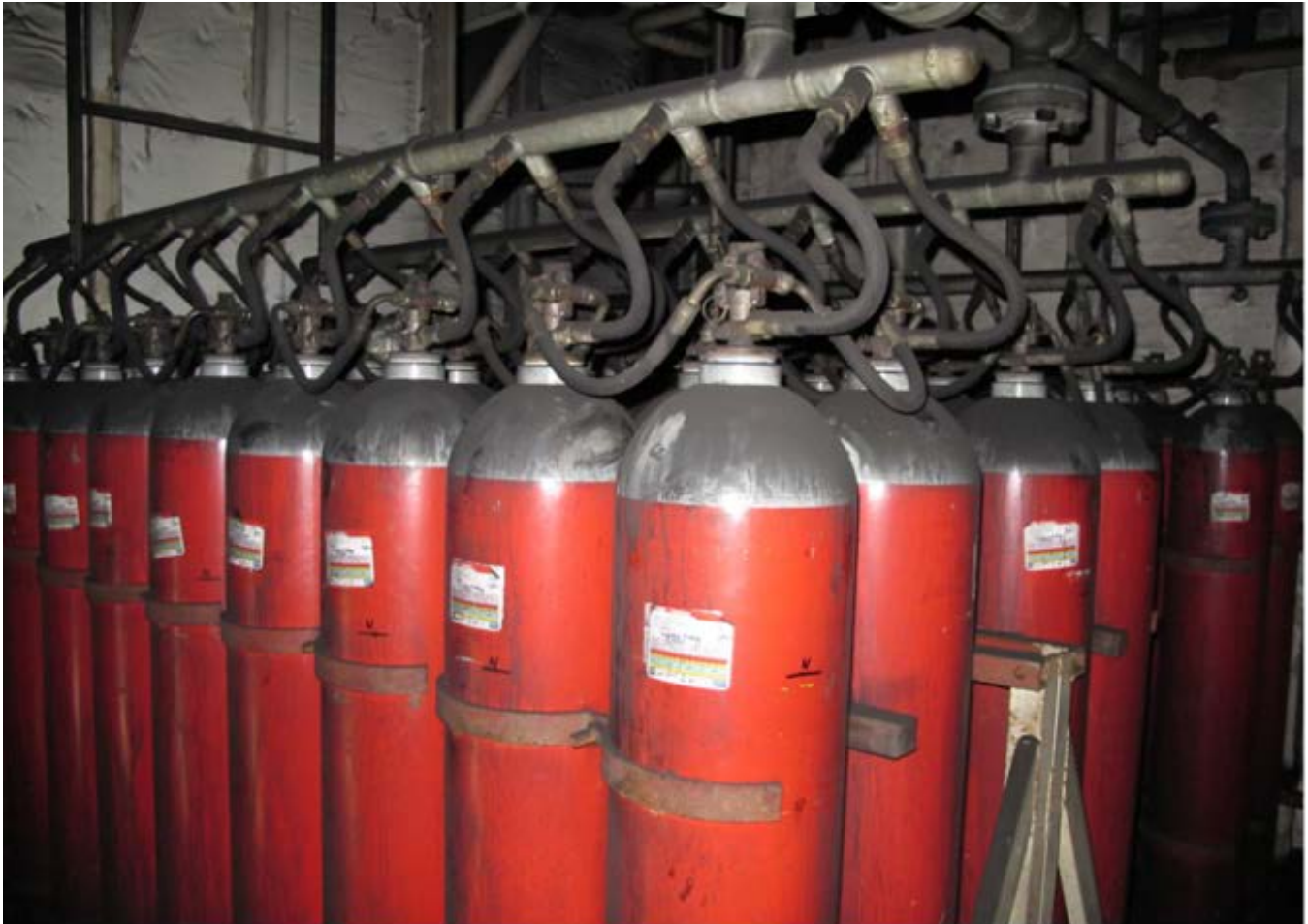
Figure 10. Photograph of upper deck of CO 2 room.
