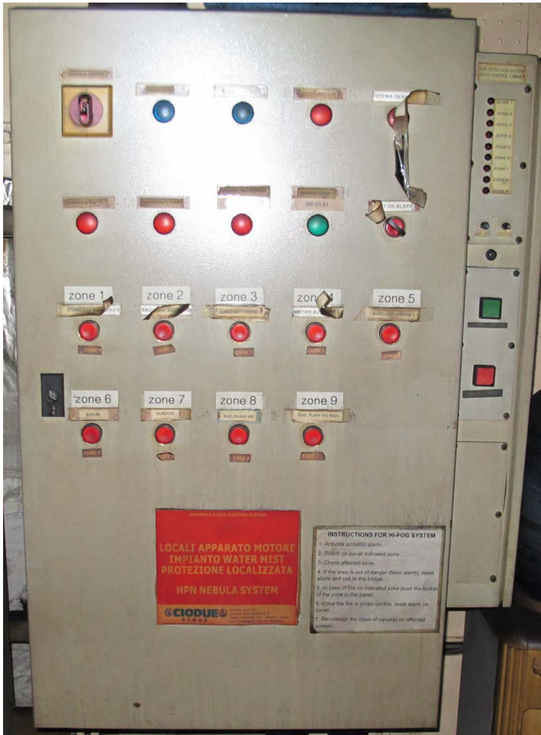
Figure 18. Photograph of water mist control panel in engine control room.
