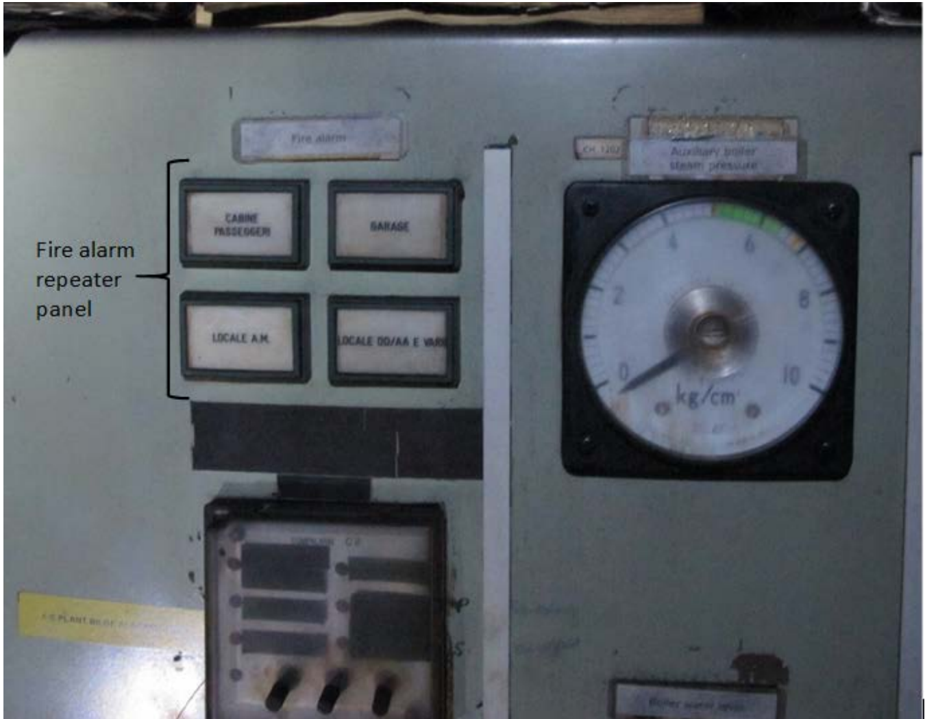
Figure 5. Photograph of fire alarm repeater panel in engine control room. Note the fire alarm repeater indicator text is in Italian.
