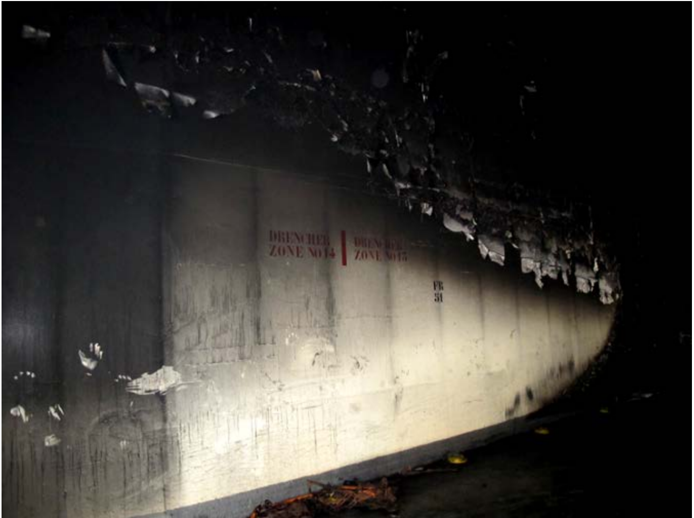
Figure 34. Photograph of forward section of damage (approximately frames 44–55) on the port side of Garage Deck B. The left side of the photograph is aft, and the right side is forward. Frame 51 and drencher zones 13 and 14 are painted on the bulkhead.
