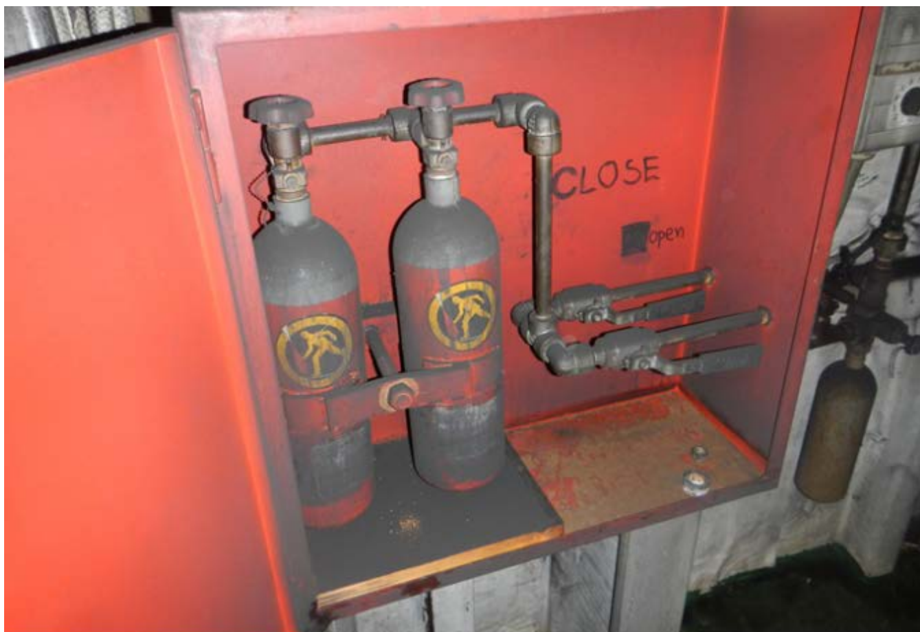
Figure 14. Photograph of interior of pilot cabinet. Both valves are in the open position.
