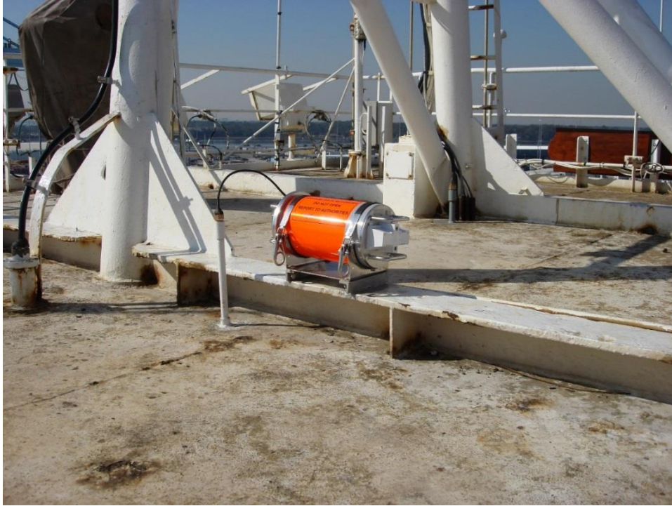
Figure 3. VDR capsule installed on El Faro’s weather deck, February 2009 (photo from Radio Holland).
