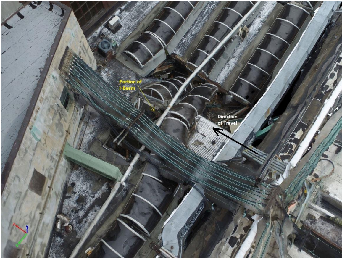
Figure 20: A photograph from the drone flyover showing the damaged canopy with glass panels and a portion of the train. The direction of train travel and a portion of the I-beam are labeled on the image.
