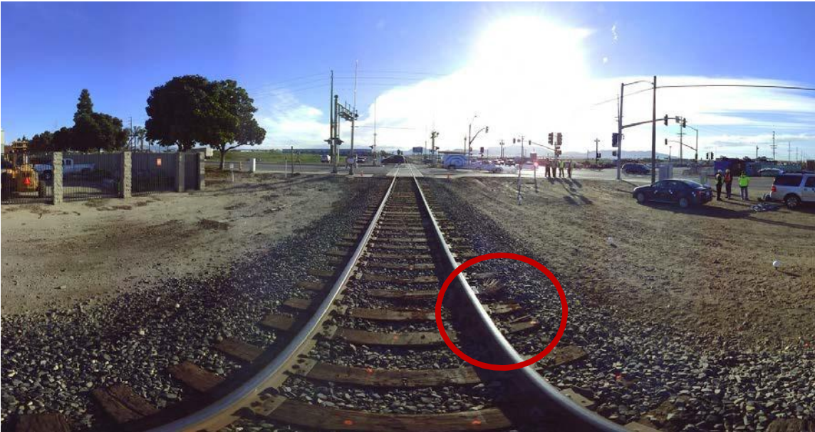
Figure 13: An image from the scanner showing the track near the point of impact. The view is looking east toward the grade crossing. The area highlighted in the red circle shows the location of the damaged railroad ties near the point of impact.
