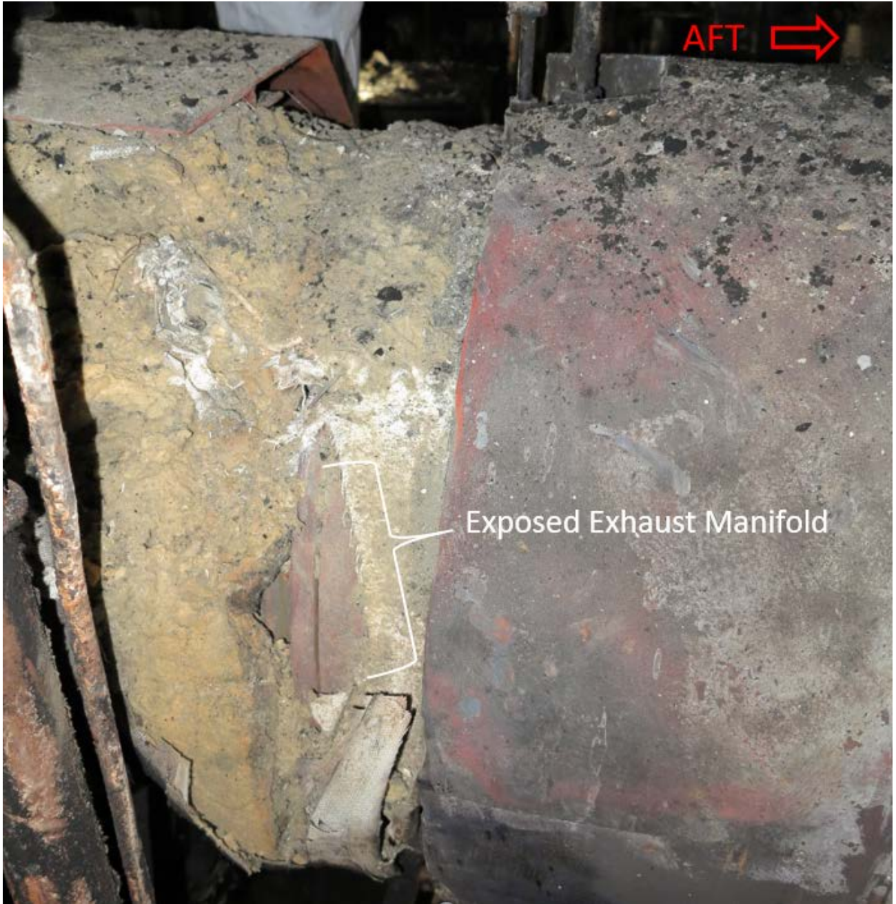
1 2 Figure 23. Caribbean Fantasy's main engine exhaust trunk with degraded insulation and exposed 3 exhaust manifold pipe. Post accident photograph of the inboard inlet side of the exhaust pipe before 4 the turbo taken from the PME drive (coupling) end.
