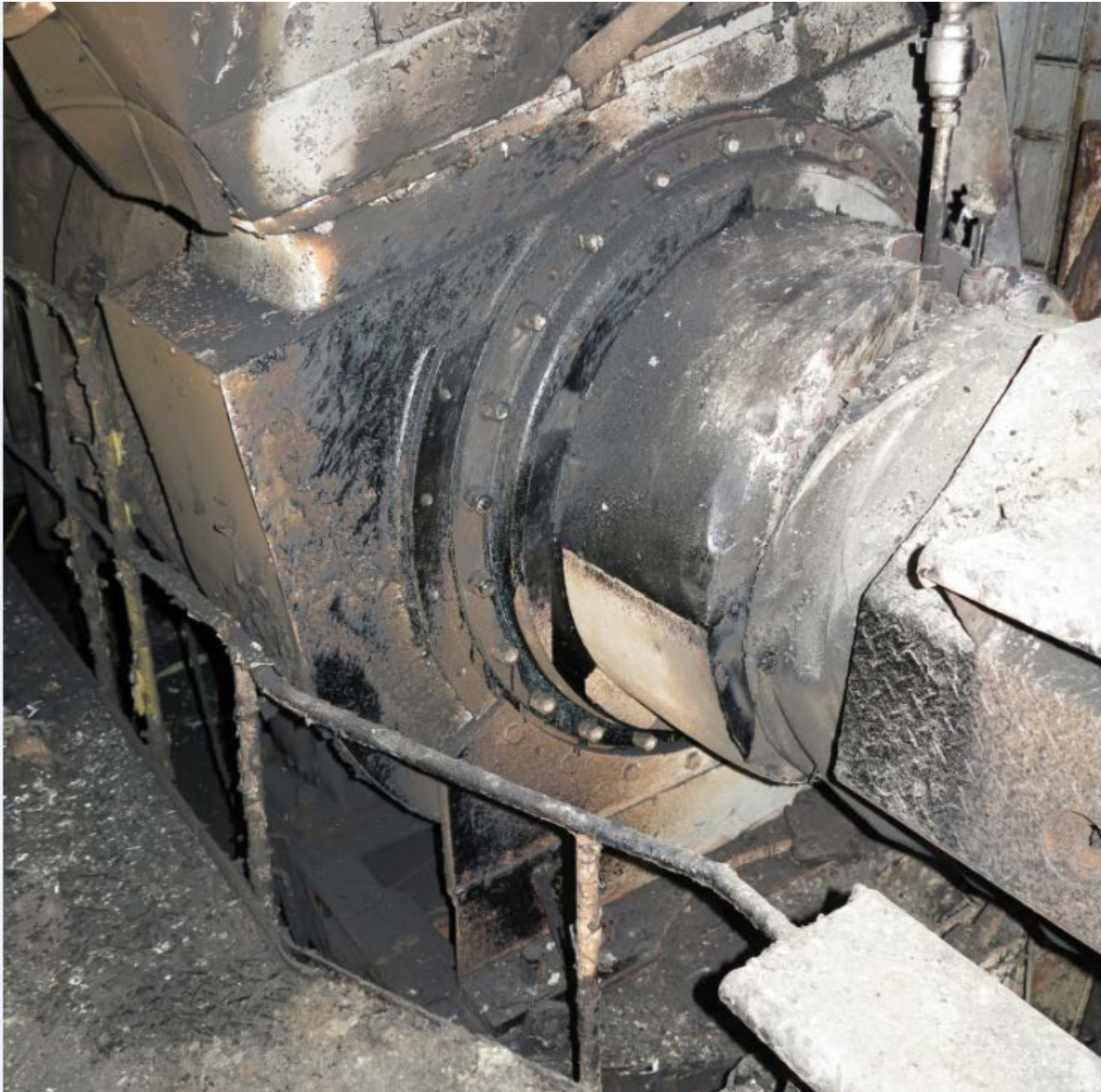
1 2 Figure 144. Caribbean Fantasy's port turbocharger casing and exhaust manifold. Dark residual oil coats 3 the forward inboard side of the turbocharger casing and exhaust manifold lagging. Postaccident 4 photograph taken from the inboard side of the PME.
