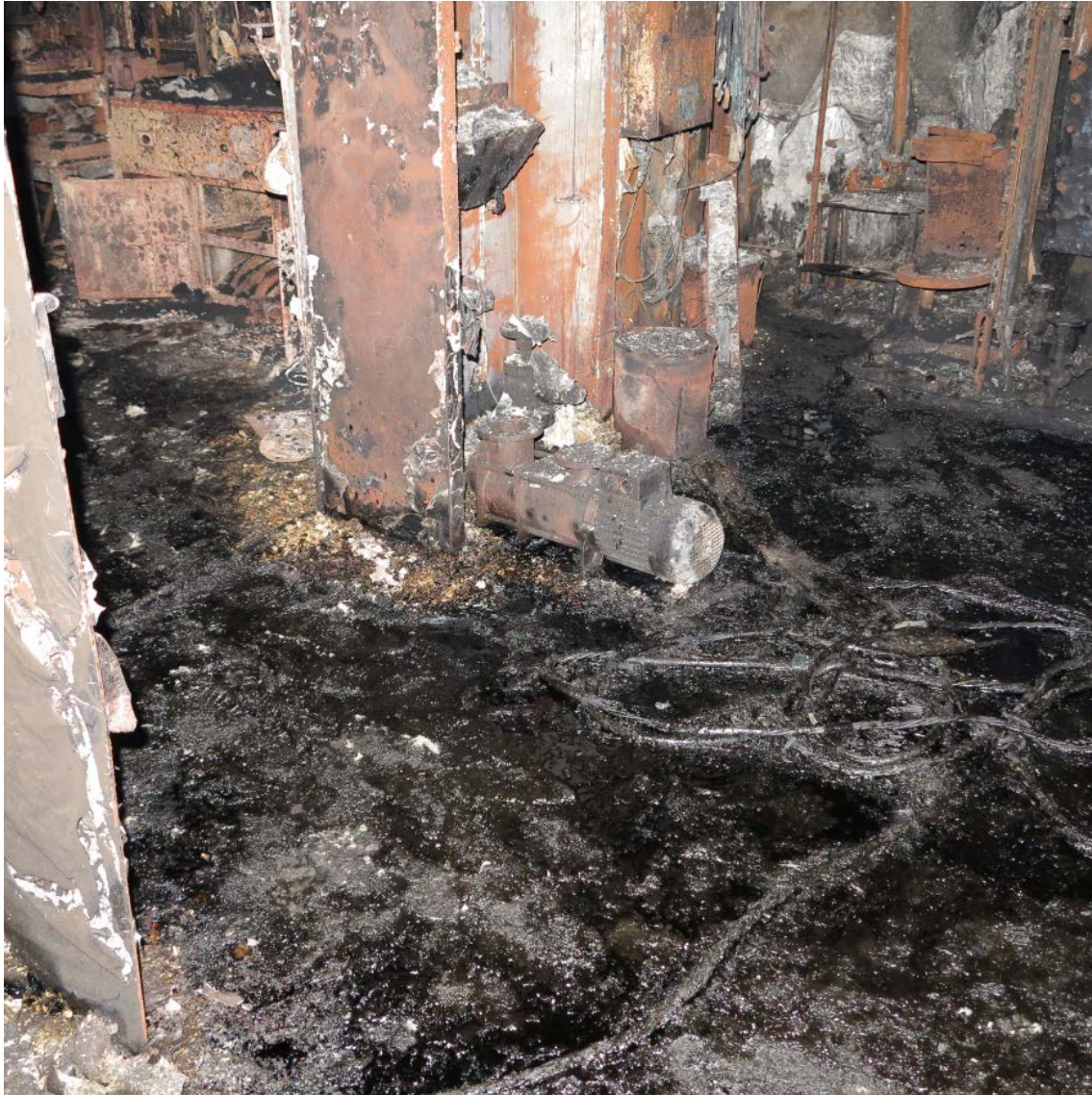
1 2 Figure 15. Port side view of the main engine room looking forward into the engine 3 workshop, deck 2, at frame 75. An inch and a half of lube oil is on the deck.
