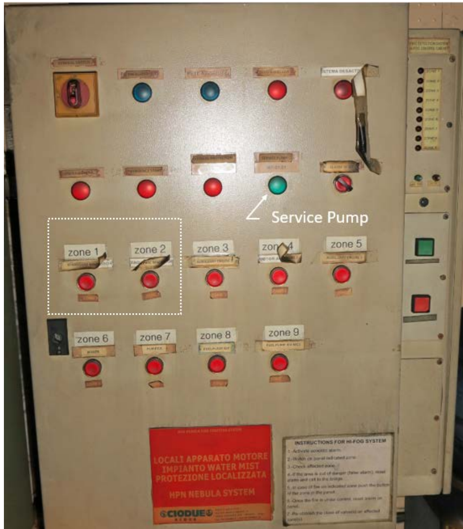
1 2 Figure 4. The HPN Nebula firefighting system localized protection system panel located in the ECR. 3 White dotted box indicates the zones the chief engineer said he activated and arrow shows the green 4 indicator light for the service pump (MP.01.01)
