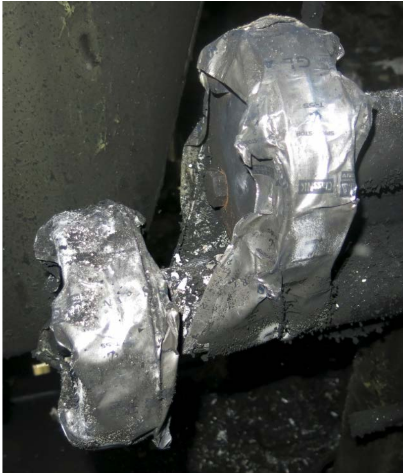
6 7 Figure 17. Caribbean Fantasy SME fuel oil supply and return line flanges and blanking plates as found 8 by investigators. Photo illustrates the wrapping of spray tape around each flange and blanking plate 9 and the classification approval stamps on the tape.
