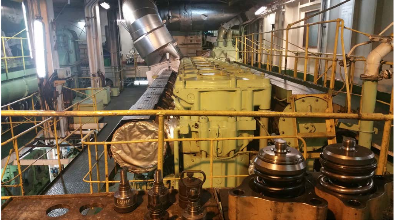
1 2 Figure 27. Caribbean Fantasy's PME photograph taken prior to the shipyard from the forward end of the 3 engine's centerline in the aft direction (inboard, exhaust manifold side of the PME).
