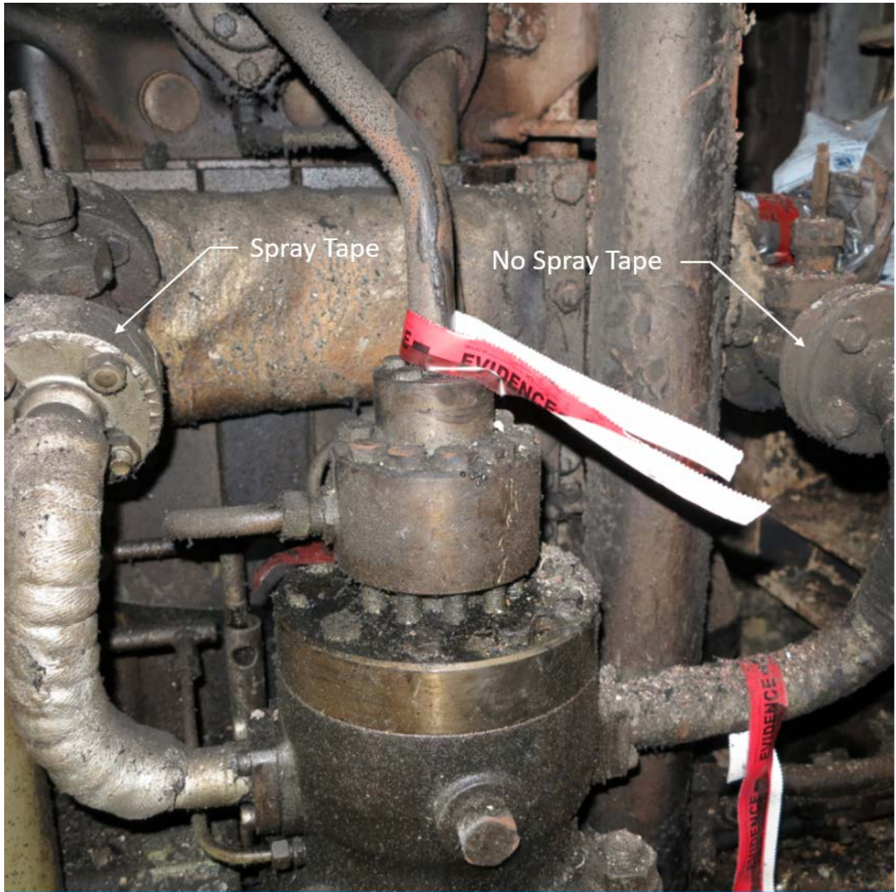
1 2 Figure 17. Caribbean Fantasy PME fuel oil supply and return line flanges on cylinder no. 8 near the drive 3 (coupling) end, lower left control side where the fuel injection pumps and the camshaft are mounted 4 (opposite to the exhaust manifold) after the fire. Photo illustrates the limited application of spray tape.
