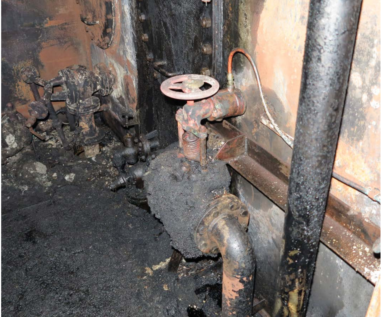
1 2 Figure 8. Caribbean Fantasy's port lube oil storage tank QCV that was intentionally blocked open. The 3 bolt and nut were removed to verify the valve stem closed.
