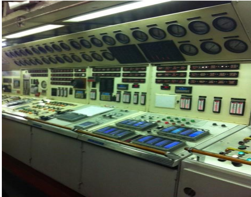
1 2 Figure 5. El Faro boiler control console (photo by Maine Maritime Academy cadet).
