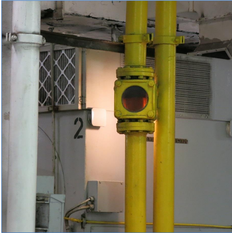
1 2 Figure 8. “Bulls-eye” for monitoring lube oil flow to main engine (photo from El Yunque ).
