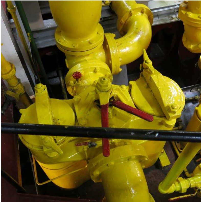
1 2 Figure 9. Lube oil service suction strainers (photo from El Yunque ).
