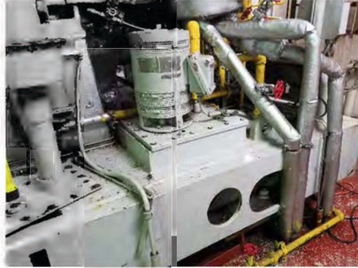
Turbo Generator Standby Lube Oil Pump Motor
