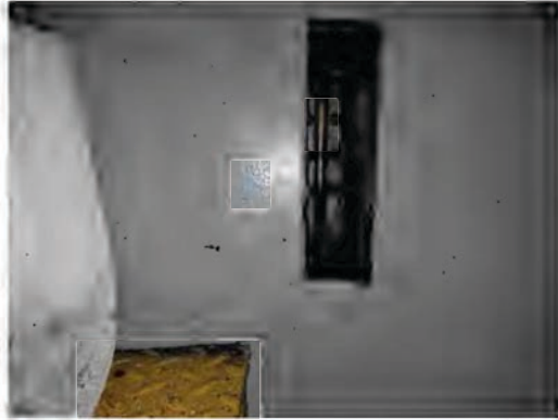
Turbo Generator Sump Lube Oil Sight Glass Mounted Vertically on the Port Side of the Sump
