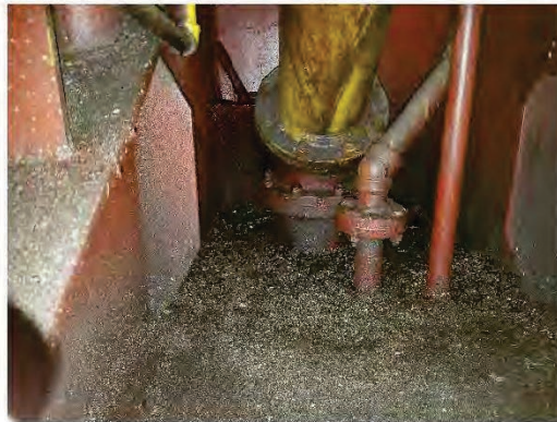
Main Lube Oil Suction Pipe at Inner Bottom
