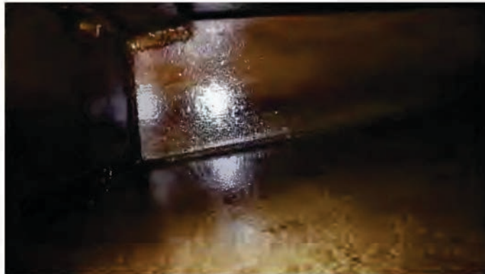
Turbo Generator After Sump Section Looking Forward. Limber Holes to the Upper and Lower Left of the Picture Drain to the Main Sump Section
