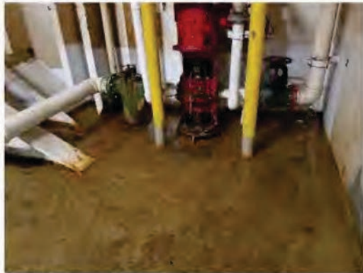
Emergency Fire Pump No. 3 Cargo Hold Port Side Aft
