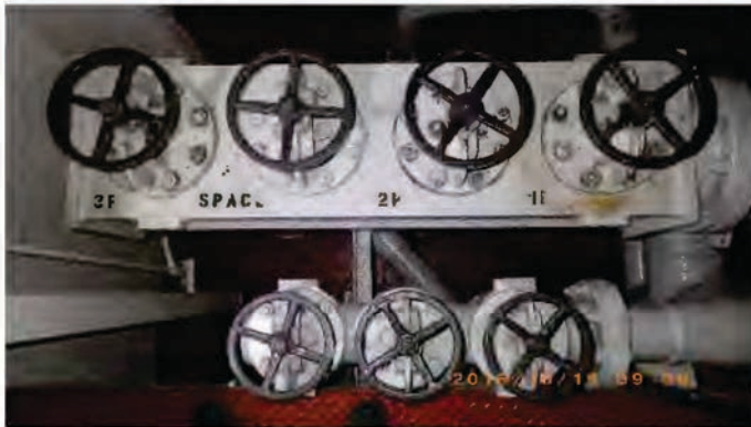
Port Cargo Hold Ballast Manifold
