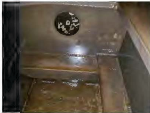
Limber Holes and Center Frame Port Side/ Center Channel/ 2 nd Bay from Aft Looking Forward
