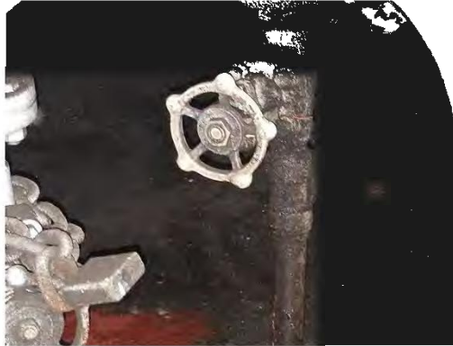
Lube Oil Storage Tank Drop Valve
