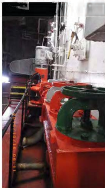
No. 2 Bilge & Ballast Pump and Suction Manifold
