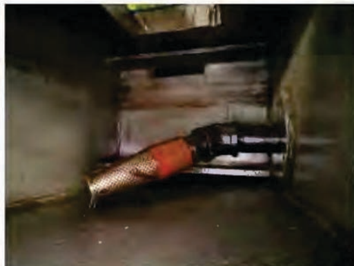
Turbo Generator Main Lube Oil Pump Suction Nozzle Viewed from Sump Looking Forward. Internal Baffle can be seen Forward of Suction Nozzle
