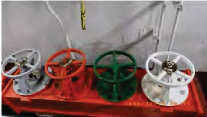
No. 2 Bilge & Ballast Pump Suction Manifold
