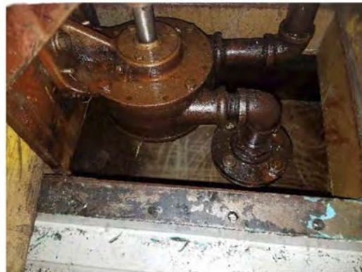
Turbo Generator Standby Lube Oil Pump and Suction
