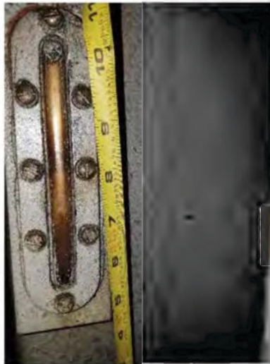
Turbo Generator Sump Lube Oil Sight Glass
