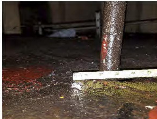
Lube Oil Storage Tank Drop Line
