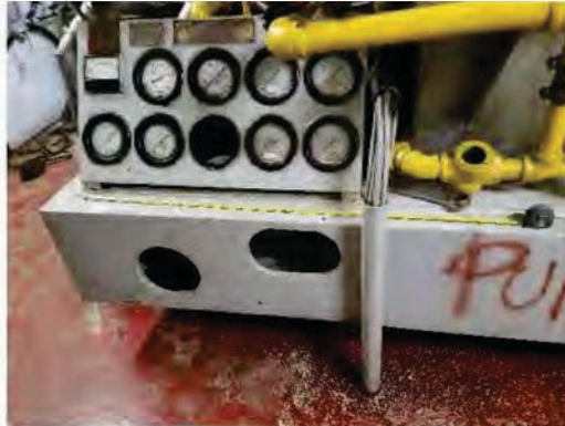
Turbo Generator Looking Forward. Measuring Tape Indicates Length of After Sump Section
