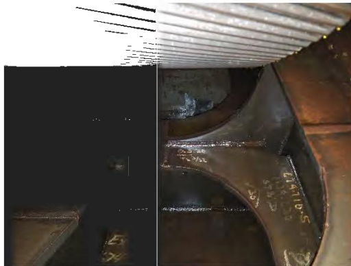
Sump Framing and Limber Holes from Port Side looking down to Center Channel
