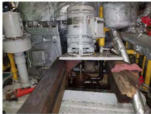
Turbo Generator Standby Lube Oil Pump and Motor
