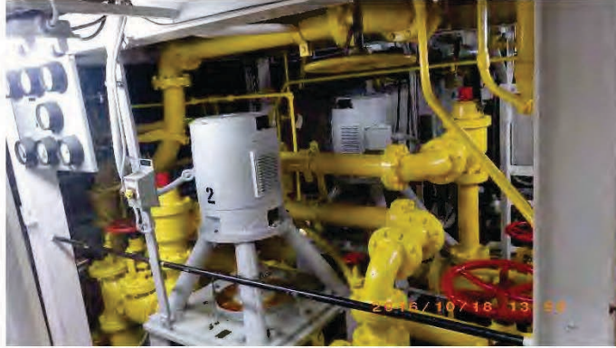
Main Lube Pumps
