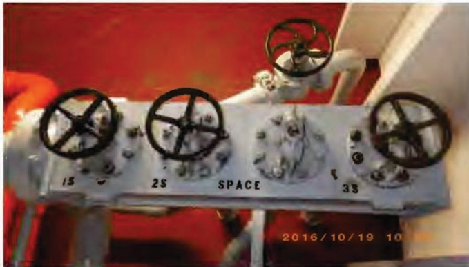
Starboard Cargo Hold Ballast Manifold
