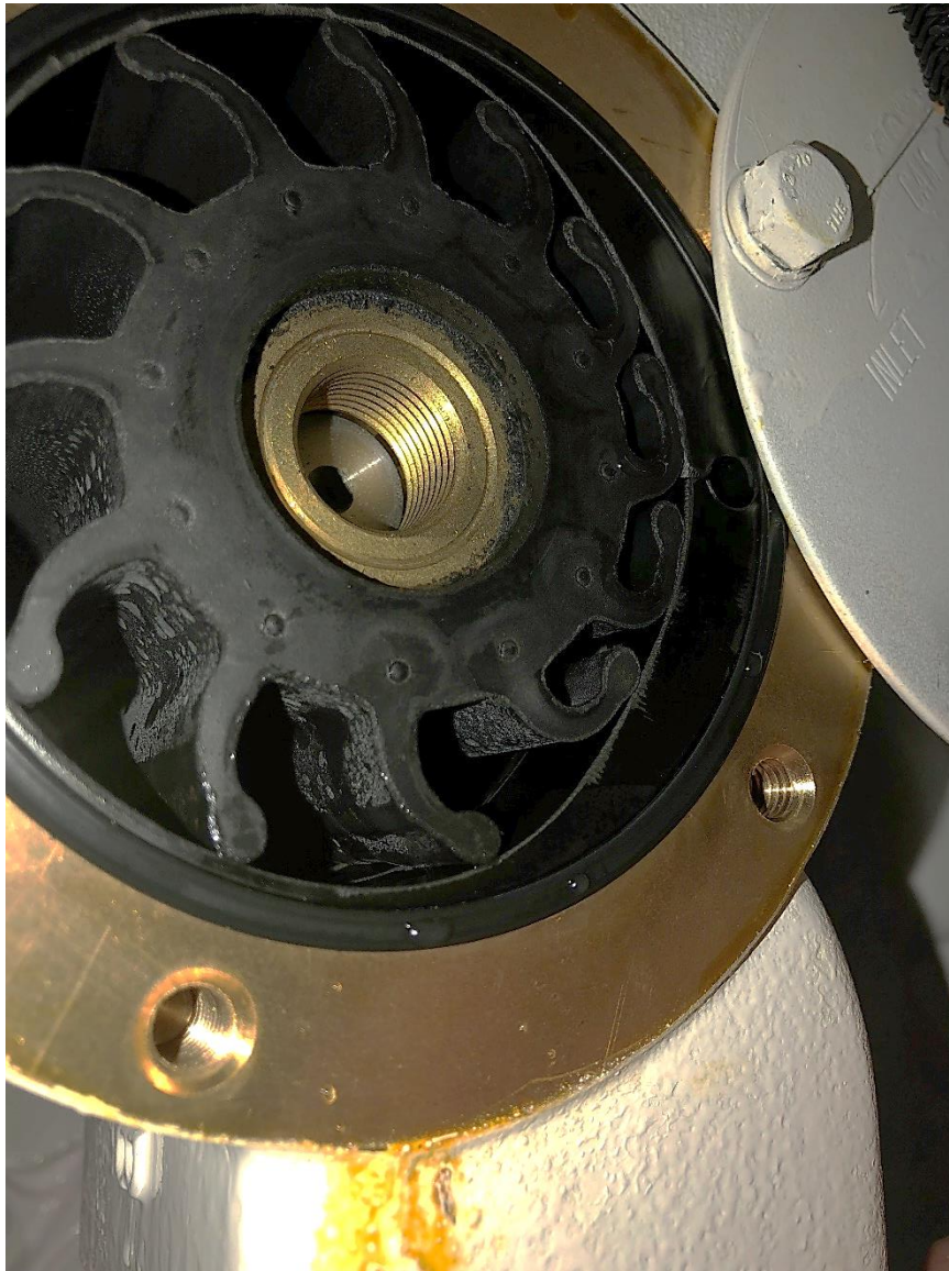
1 2 Figure 22. New raw-water pump impeller installed in its pump housing. (Photo provided by 3 Ring Power) 4
