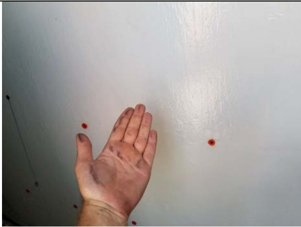
Interior covered with fine black soot (wipetest failed)
