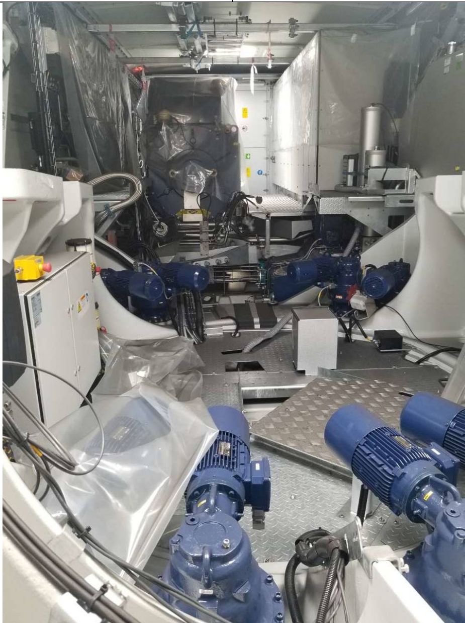
View inside nacelle
