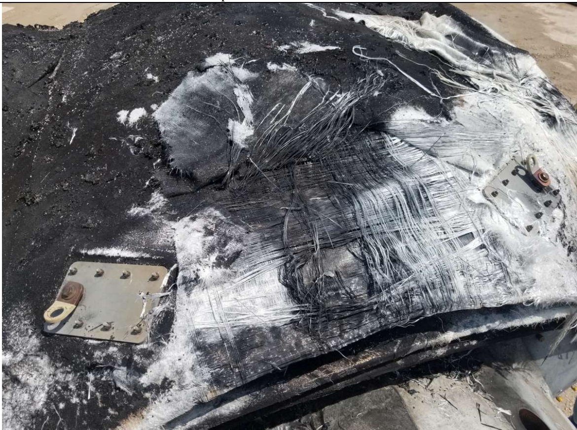
View onto top of burnt hub #18020106 at Free Trade Zone during inspection
