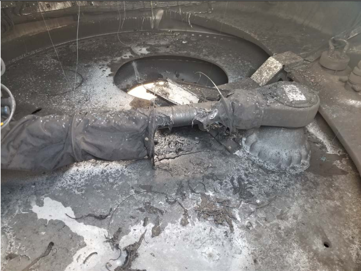
View inside burnt hub #18020106
