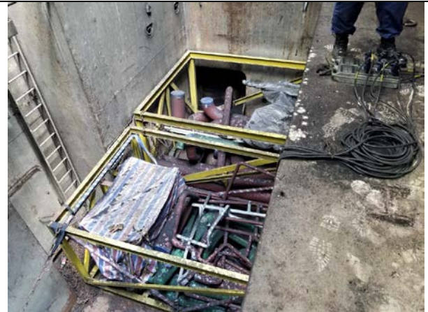
Entrance to lower hold obstructed by construction parts
